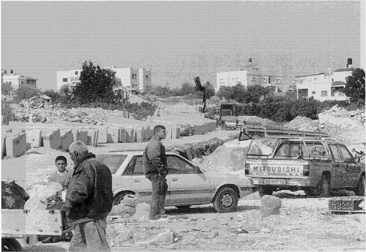
Photograph 11: Nazlat Issa, Tulkarem Governorate (24 November 2003): After the destruction of the market in August 2003, the rubble was cleared and Israelis prepare to erect the 8 - meter high concrete Wall encircling the Palestinian towns of Baka Sharqiya, Nazlat Issa and Abu Nar, in effect destroying the economic viability of this once thriving market hub.
