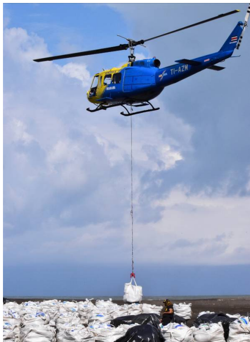
Photo 3. Partial view of the work of hooking the sacks for transport at the mouth of Agua Dulce Lagoon. Photo by Miguel Araya, 4 April 2015.
