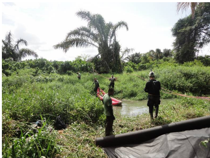
Photo 4. Partial view of site selected for construction of the dyke. 30 March 2015 Photo by Christian Birkel.
