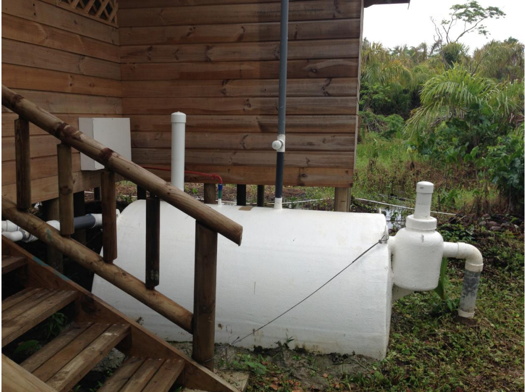
Figure 13: Sewage treatment plant of the MINAET biological station
