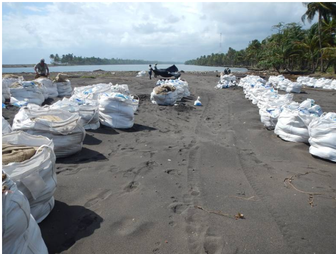
Photo 12. Partial view of the sack filling area after the works were completed. Photo by Miguel Araya, April 08, 2015.
