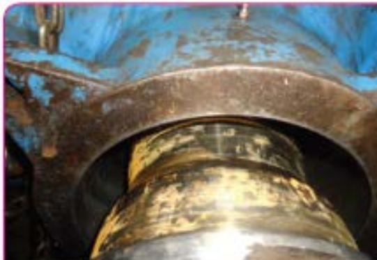
"SOBERANÍA I" worn-out pump bushing
