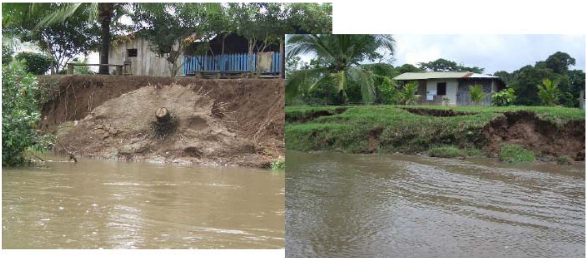
Collapse of the riverbanks:
