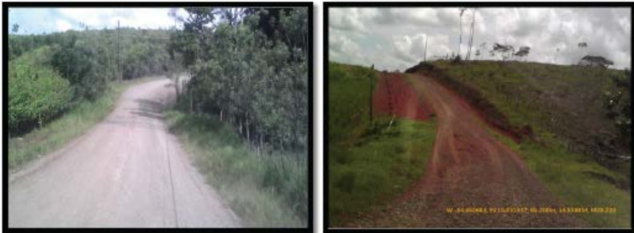
F20. Lack of maintenance to the drainage canals.
