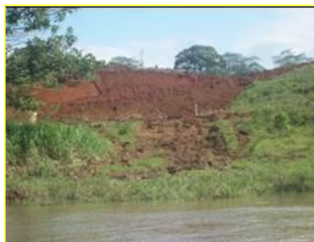
Figure 14: Cross-section of inadequately sloped embankment
