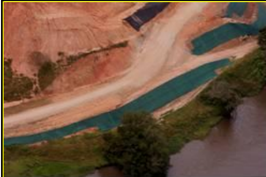
Figure 39: Critical point due to slope instability and ongoing erosion process
