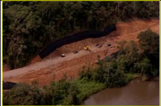
Figure 42: Critical point due to slope instability
