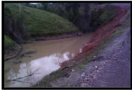
F34. Stagnant water with no drainage whatsoever.
