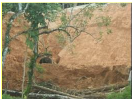
Figure 13: Culvert with a smaller diameter than recommended
