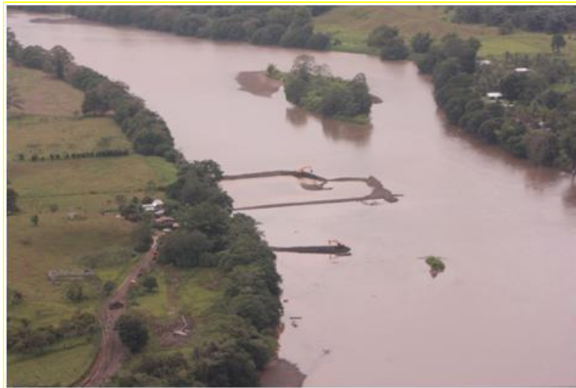
Figure 4: Embankments to build a bridge over the San Carlos River Source: FUNDENIC, February 11, 2012.
