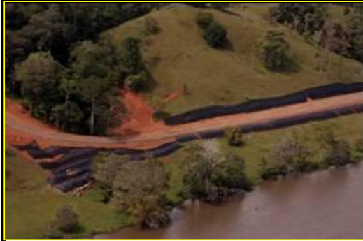
Figure 41: Critical point due to sediment runoff to river
