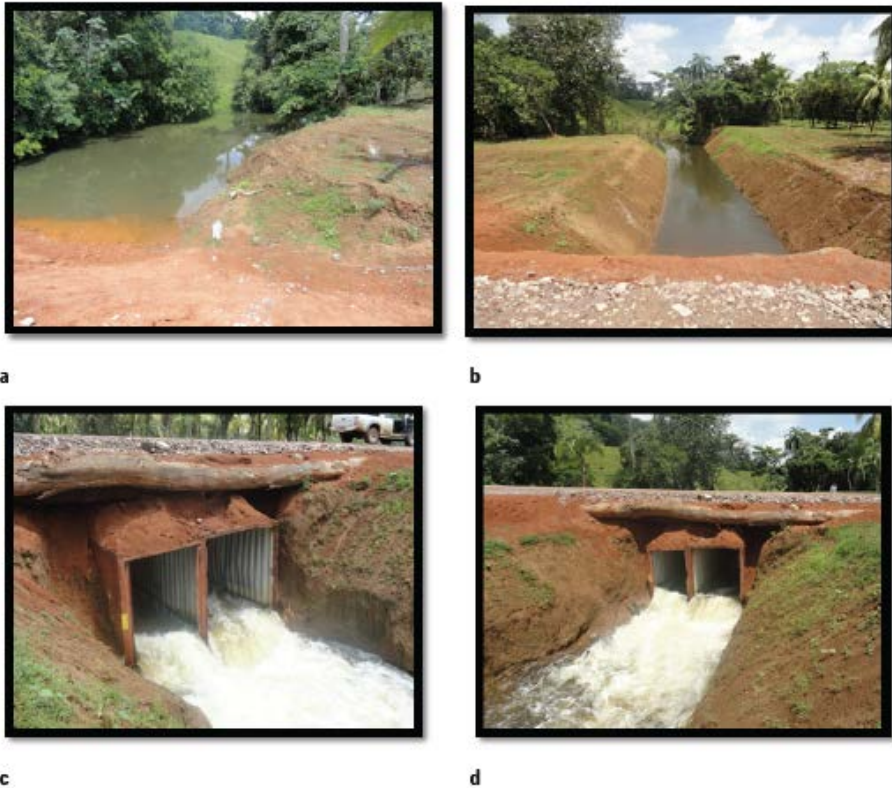
F17. Evident in the first photo (a) is the obstruction of the natural flow of the river; the second photo (b) shows the construction of a canal for re-routing the flow of the river; the last two photos (c and d) show the construction of a bridge where wooden logs and two container trailers used for drainage are part of the structure; bulging can be seen; bulging in the walls of the container trailers can also be seen.
