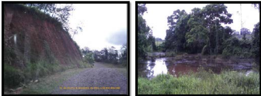
F22. Slope approximately six meters in height with an almost vertical slope.
