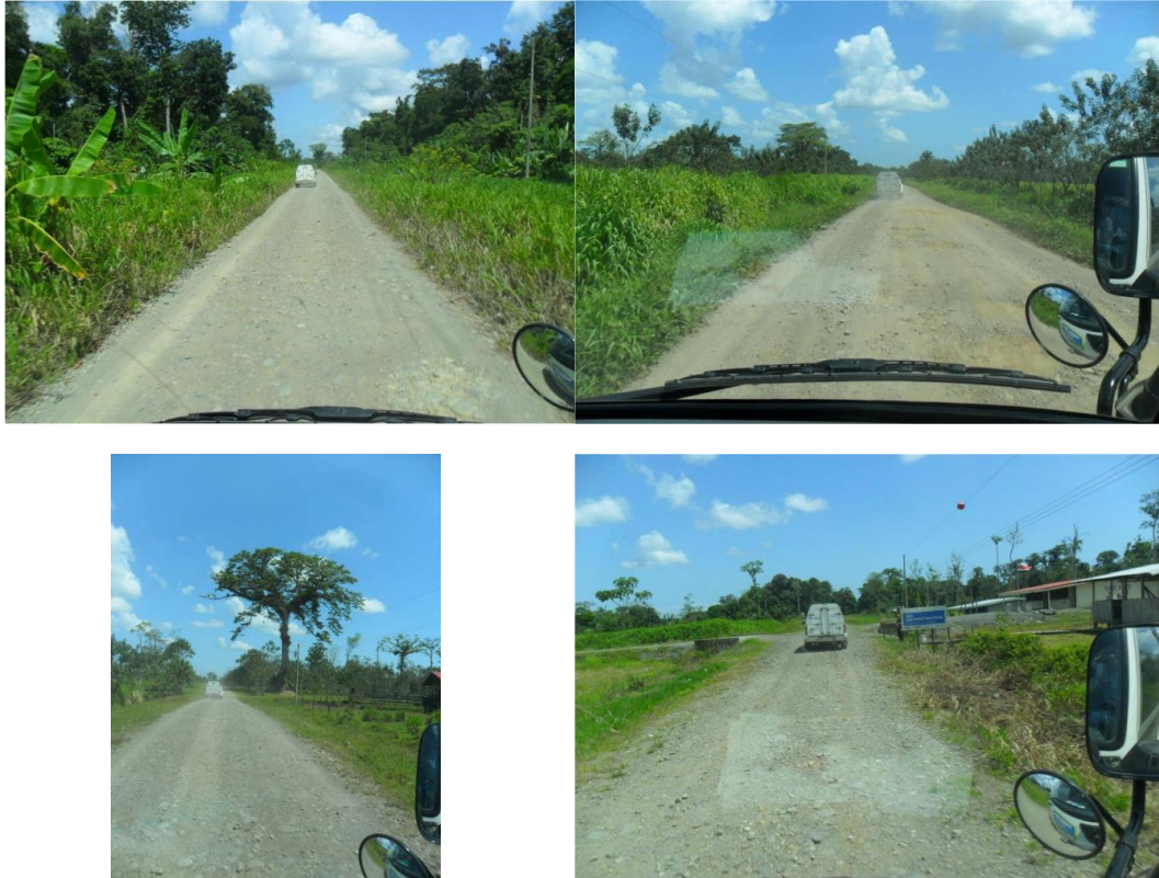
Figure 2. Photographs representative of conditions observed by the author along the Road between Boca Sarapiquí and the Delta on the ground on February 16, 2013.
