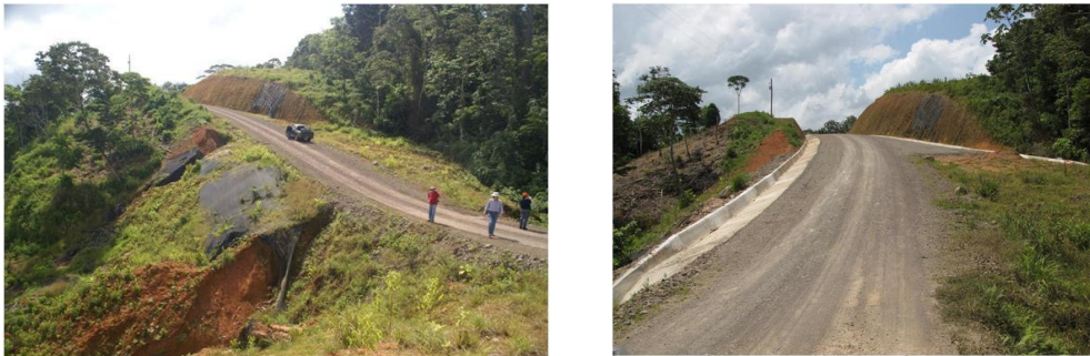
Figure 41. Road at East 497867, North 325463 about 6.4 km east of Marker II (a) on 15 February when failure of geotextile slope protection had allowed concentrated out-board runoff from the Road to create two gullies and in-board runoff was undercutting a cut slope (b) on 7 May 2013 after construction of concrete-lined out-board and in board ditches.
