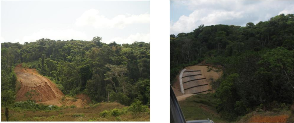
Figure 44. Path cleared for the Road near Crucitas, just east of the Rio Infiernito (a) on 15 February when unmanaged runoff from the path cleared in preparation for construction of the road bed had caused sheet and rill erosion. (b) The same area on 7 May 2013 after installation integrated measures to manage runoff involving regrading, silt fences, and concrete-lined outboard ditch. Photographs by author.
