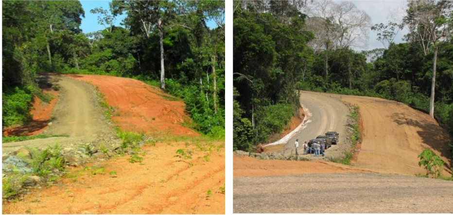
Figure 2.3 The Road near Marker II (a) prior to mitigation work on 15 February 2013 and (b) on 7 May 2013 with mitigation measures in place. 119
