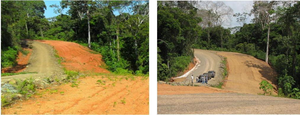
Figure 39. The Road near Marker II (a) prior to mitigation work on 15 February 2013 and (b) on 7 May 2013 with mitigation measures in place: note in-board drainage channel and extensive biodegradable, erosion control matting. Photographs by author.
