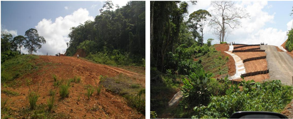
Figure 2.4 Road at East 502480, North 321561, close to the Río Infernito (a) on 15 February 2013, and (b) the same stretch of road on 7 May 2013. 120
