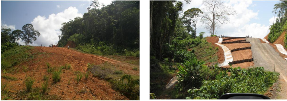
Figure 43. Road at East 502480, North 321561, close to the Río Infiernito (a) on 15 February when surface unmanaged runoff from the road bed and surrounding slopes disturbed during construction had caused sheet and rill erosion of bare soil surfaces. (b) The same stretch of road on 7 May 2013 after protection of the road surface using crushed rock, installation of silt fences to prevent sheet and rill erosion while directing down-slope surface runoff into concrete-lined outboard and inboard ditches. Photographs by author.
