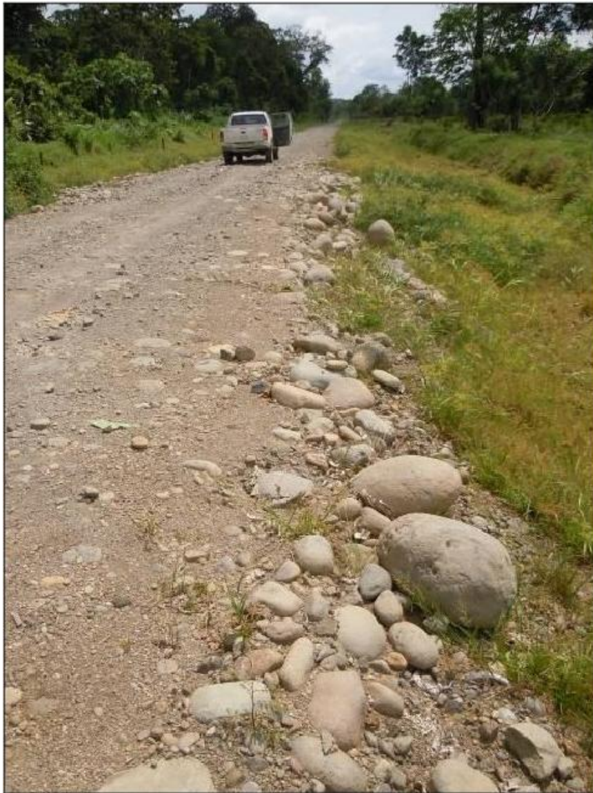
Figure 9. Current platform condition, road section 2. Source: LanammeUCR, May 2012
