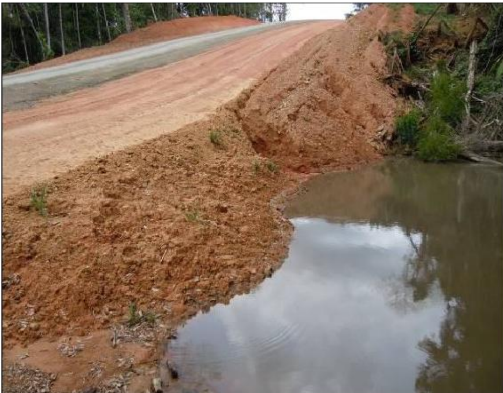
Figure 33. Blocked bodies of water. Source: LanammeUCR, May 2012
