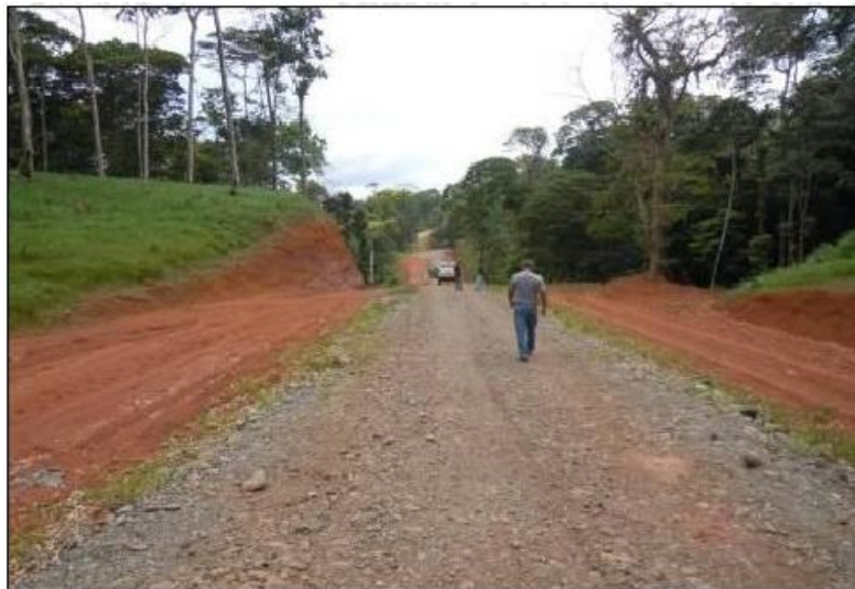
Figure 12. Nonexistent side drainage structures. Source: LannameUCR, May 2012
