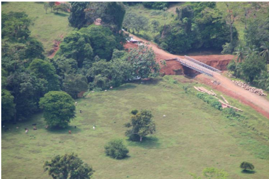
Figure 23. Photo of bridge being constructed across Cano Curenita about 58 km downstream from the upstream end of Route 1856 along border. Bridges are appropriate for this larger stream, however significant volumes of sediment are being delivered to the Río San Juan as a result of construction activities including extensive ground disturbance, sidecasting and perching oversteepened fill over the stream, and the lack of surface erosion control measures.
