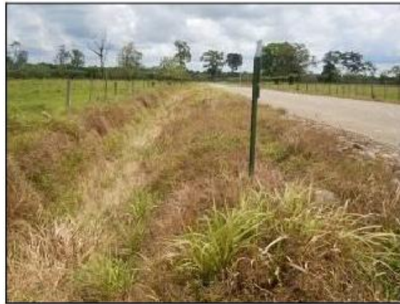
Figure 4. Condition of gutters in road section 1. Source: LannameUCR, May 2012
