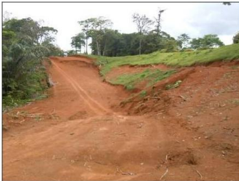
Fig. 18. Landslides in the Route, road section 4 Source: LannameUCR, May 2012
