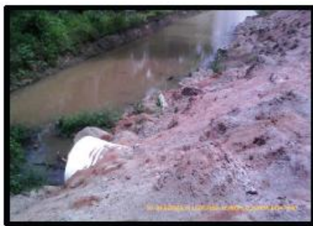
F41. Circular pipe serving as outlet for river water.
