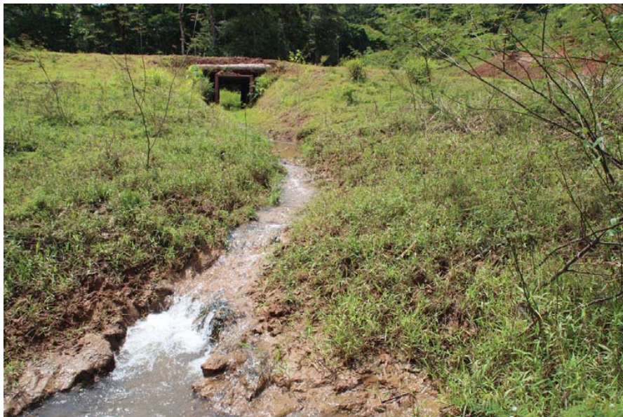
Figure 19. Photo #95e at km 21.75 from upstream end of Route 1856 along border. Use of logs as headwalls and other inappropriate crossing materials will increase the failure potential of the drainage structure and result in additional sedimentation to the Rio San Juan.
