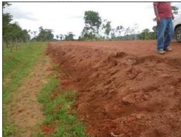
Figure 15. Fill with evidence of material sliding down from platform, road section 3 Source: LannameUCR, May 2012
