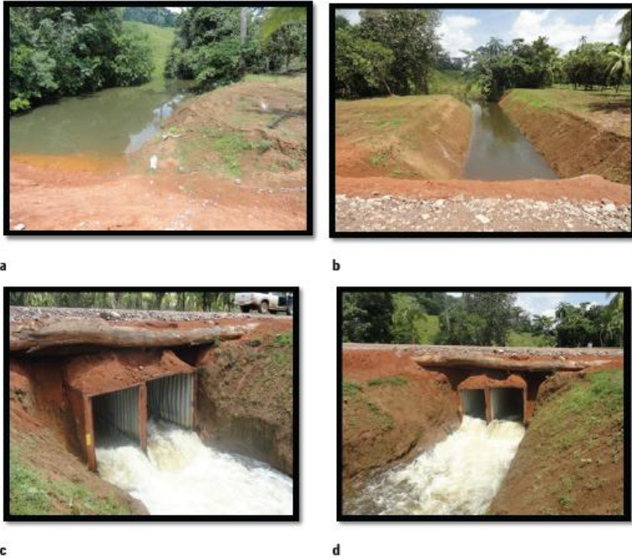
F17. Evident in the first photo (a) is the obstruction of the natural flow of the river; the second photo (b) shows the construction of a canal for re-routing the flow of the river; the last two photos (c and d) show the construction of a bridge where wooden logs and two container trailers used for drainage are part of the structure; bulging can be seen; bulging in the walls of the container trailers can also be seen.
