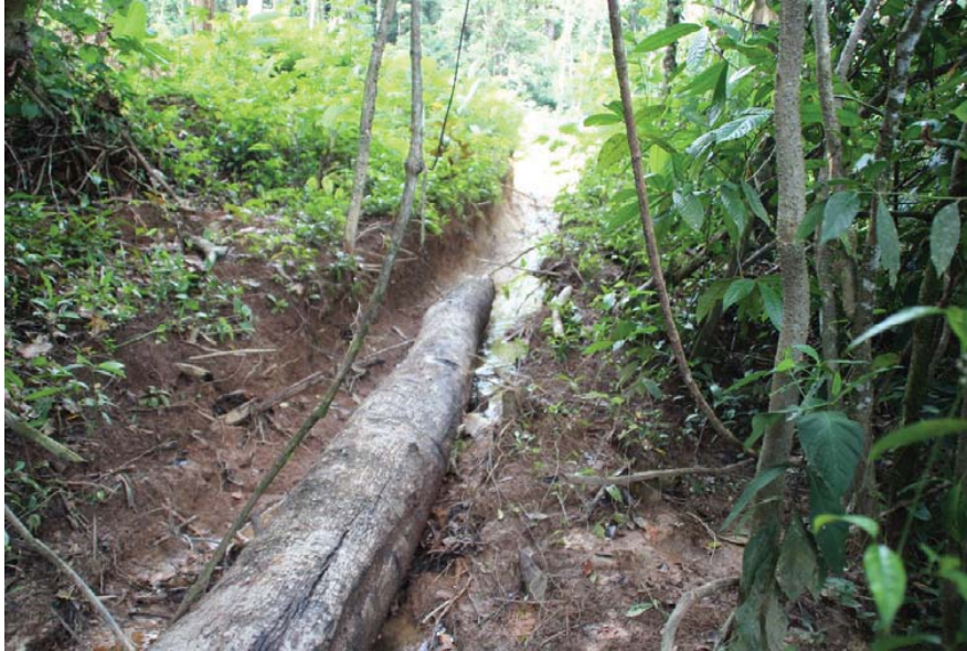
Figure 22. Photo #51c at km 11.3 from upstream end of Route 1856 at border. Road and culvert (not visible) are in the distance in the sunlight. Man-made ditch has been constructed to convey runoff to the Río San Juan where the photo was taken. Note the poor design and oversteepened sideslopes to the ditch.
