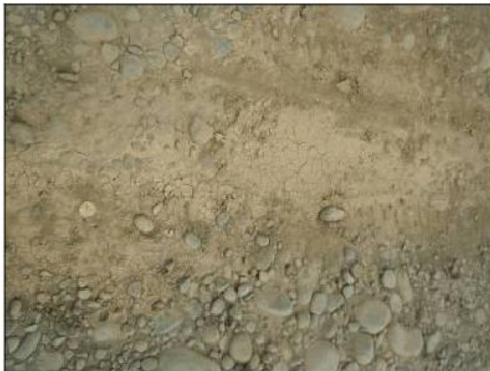
Figure 8. Holes and material contaminated with subgrade.
