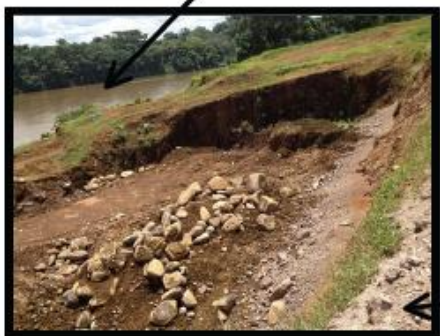
F19. Materials used are only meters away from the Río San Juan; very big boulders can be observed as well as piles of broken boulders. Here, what is apparently a trench is located between the Río San Juan and the road, several meters from the river. These situations should be evaluated.
