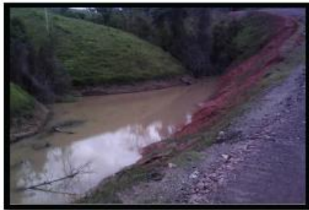
F34. Stagnant water with no drainage whatsoever.
