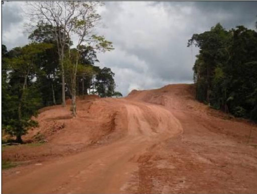
Figure 17. Sector without intervention, high ground water levels, road section 3. Source: LanammeUCR, May 2012
