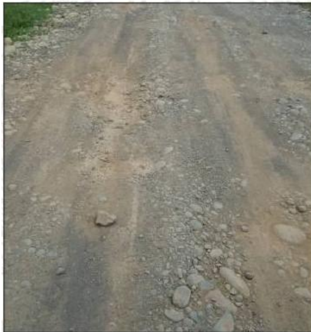
Figure 7. Deformations and contaminated granular material Source: LanammeUCR, May 2012
