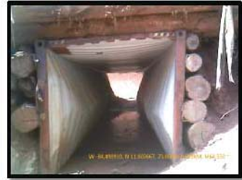
Figure 18. Photo from CFIA report dated June 2012. Stream crossing built with non-conventional materials are already failing and delivering sediments to tributary streams during every rainfall and runoff event. It is also likely the drainage structure is not properly sized for 50- or 100-year discharges.
