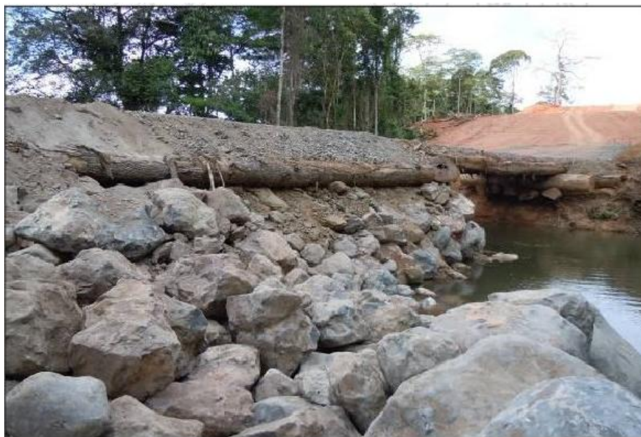
Figure 32. Log bridge over Infiernito River. Reduced hydraulic cross-sectional area. Source: LannameUCR, May 2012
