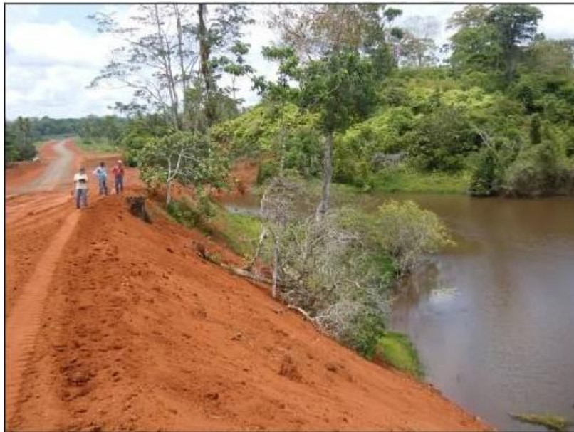
Figure 21. Inadequate cut material and embankment management. Source: LannameUCR, May 2012
