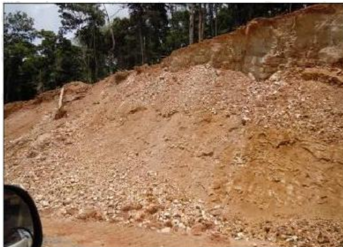
Figure 42. Slope landslides in cut areas, road section 8. Source: LannameUCR, May 2012
