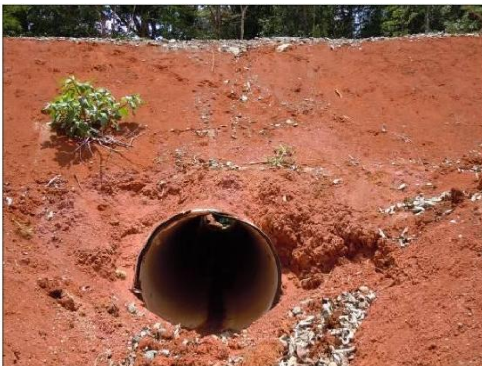
Figure 45. Poorly installed Rib-Loc pipes.
