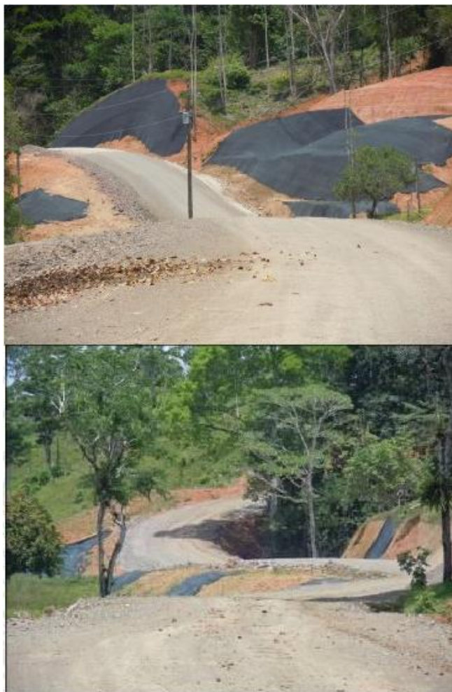
Figure 38. Saran fabric placed on cut and fill slopes, road section 8. Source: LanammeUCR, May 2012
