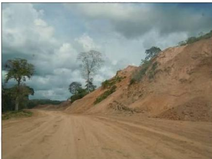
Figure 27. Unstable cut embankment, road section 6. Source: LanammeUCR, May 2012
