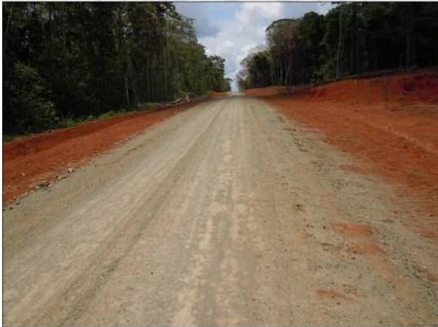
Figure 44. Inadequate road surface granular material on section 9. Source: LannameUCR, May 2012
