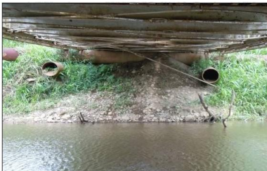
Figure 6. Bailey bridge supports in Fátima-Sarapiquí River Mouth road section. Source: LannameUCR, May 2012
