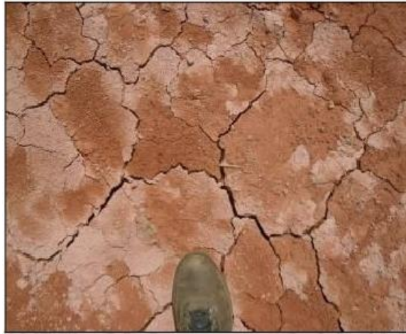
Figure 14. Soil cracking, road section 3 Source: LannameUCR, May 2012
