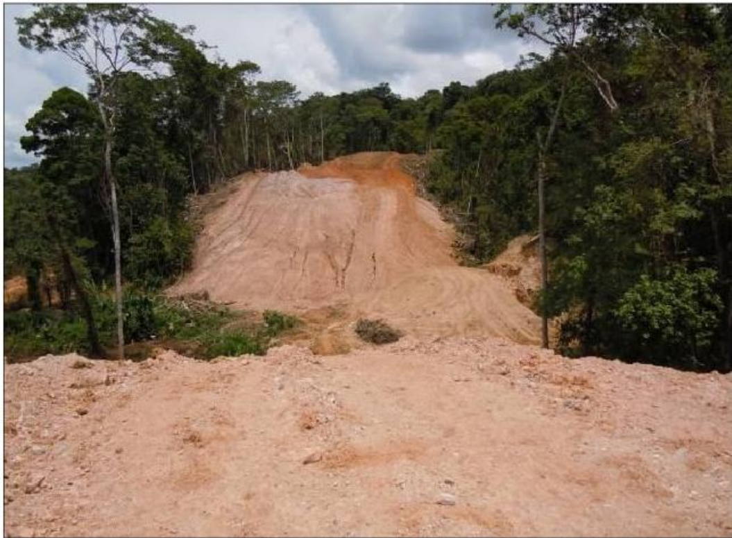
Figure 31. Cut and fill area in mountainous zone, road section 6. Source: LanammeUCR, May 2012
