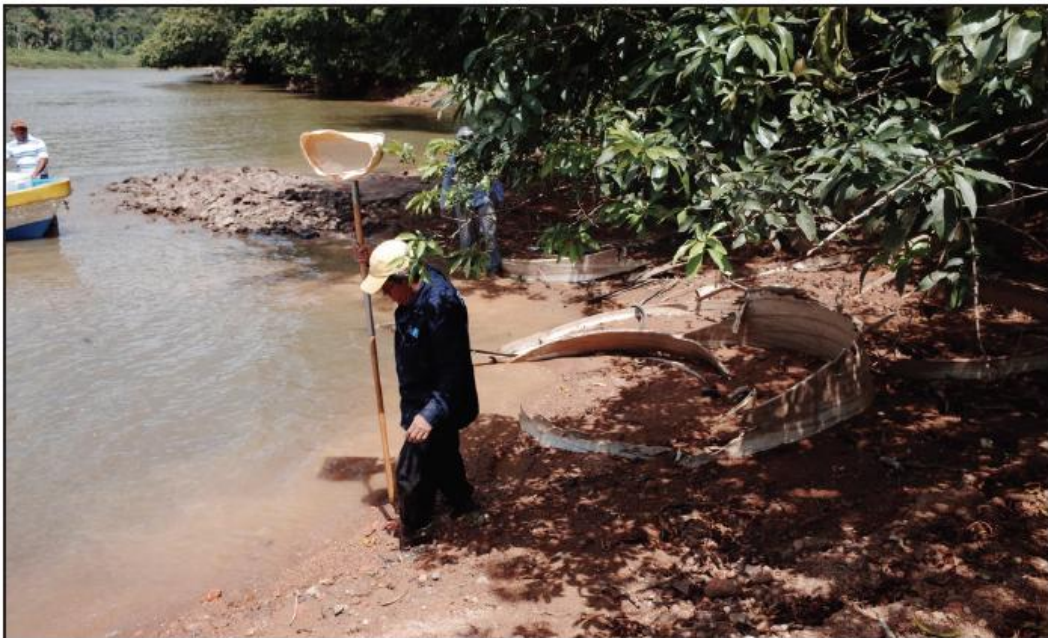
Figure 2.13. Broken culvert pipes and fill material extending into the San Juan River at location of stream crossing failure on flat land. Photograph from March 31, 2014.
