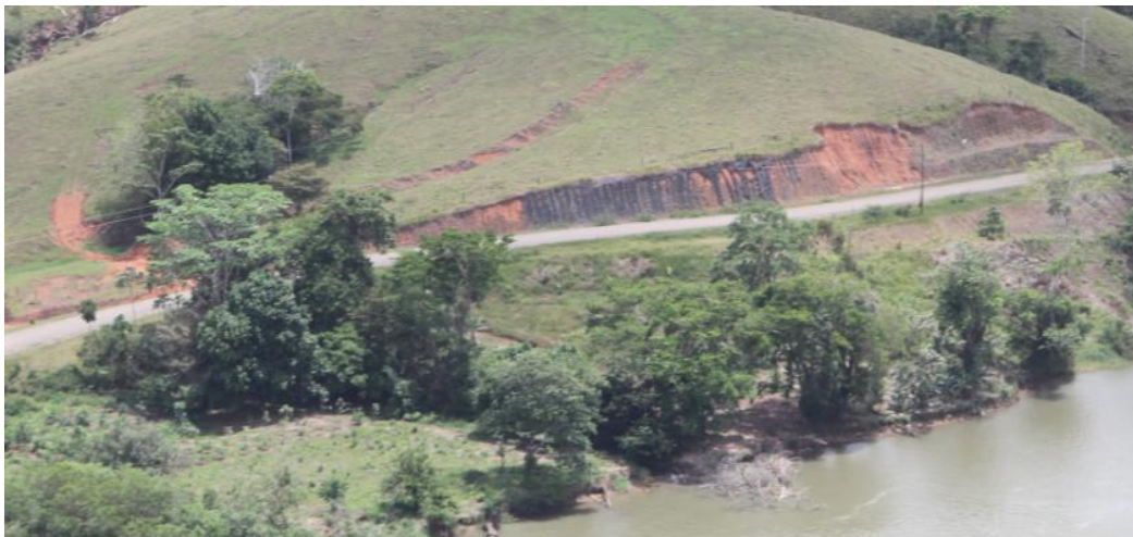
Figure 3.2. Failing geotextiles approximately 6.8 km downstream from Mojon II.
