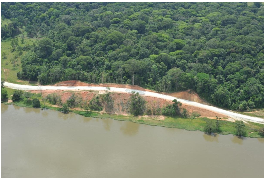
Figure 5.1. Severely Eroding Site 4.1, located 8.2-8.7 km downstream of Mojon II.
