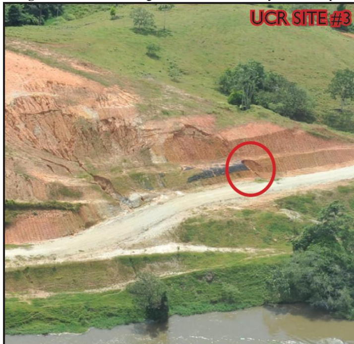
Figure 2.36. Aerial image of UCR Site 3: Gully on cut slope.
