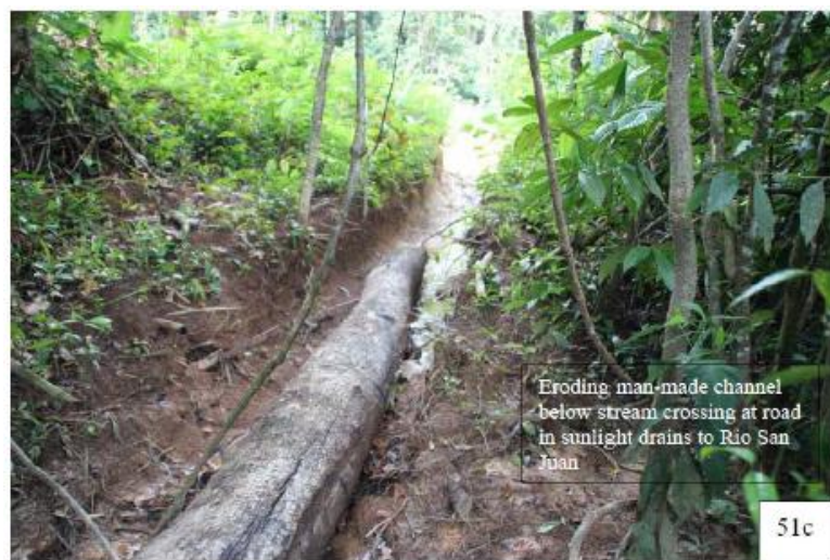
Figure 2.29. Eroding man-made channel connecting the Road to the River, located approximately 11.3 km downstream from Mojon II. Photograph from 2012 Kondolf Report, Appendix B (October 2012).
