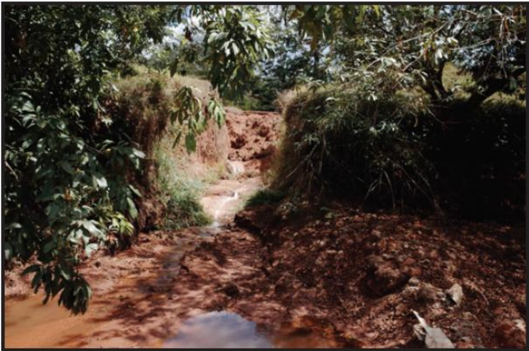
Figure 2.14. Fill placed in channel with no culvert to provide temporary crossing, allowing water to flow over the fill. Photograph from March 31, 2014.
