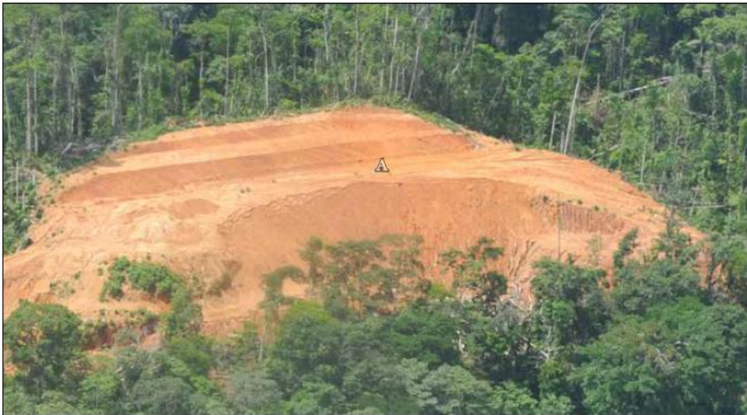
Figure 2.15. Severely Eroding Site 8.1, 16.1 km downstream of Mojon II. Oblique aerial view from October 2012.
