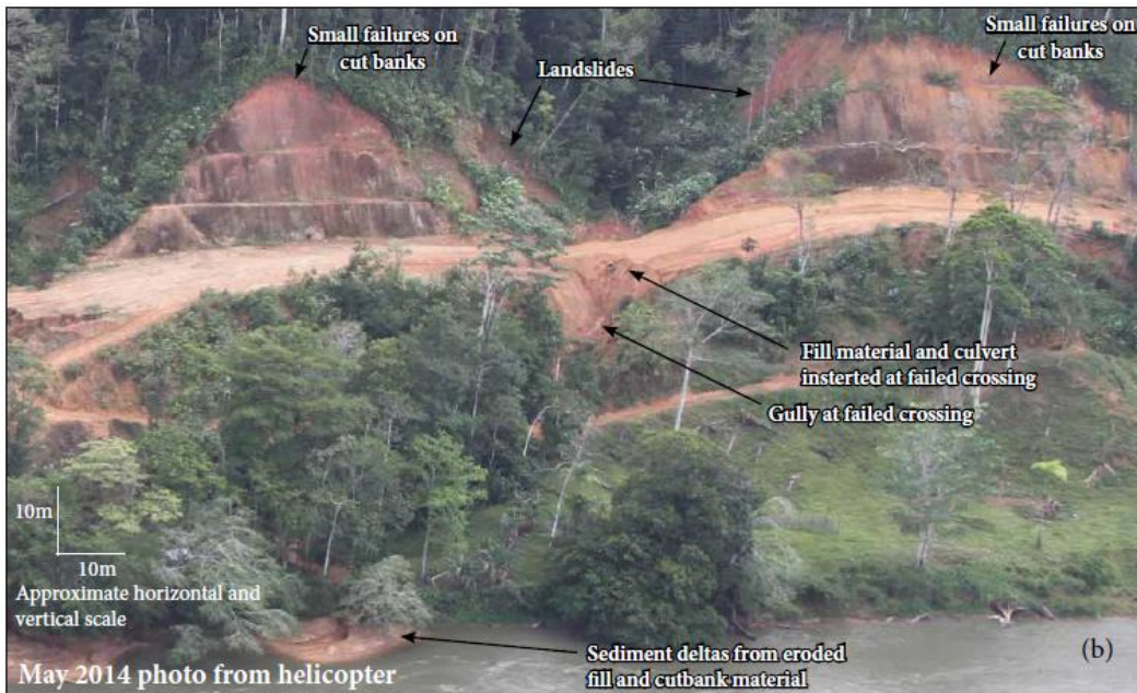
Figure 2.8. Severely Eroding Site 9.5, 18.1 km downstream of Mojon II. Oblique aerial view from May 2014.
