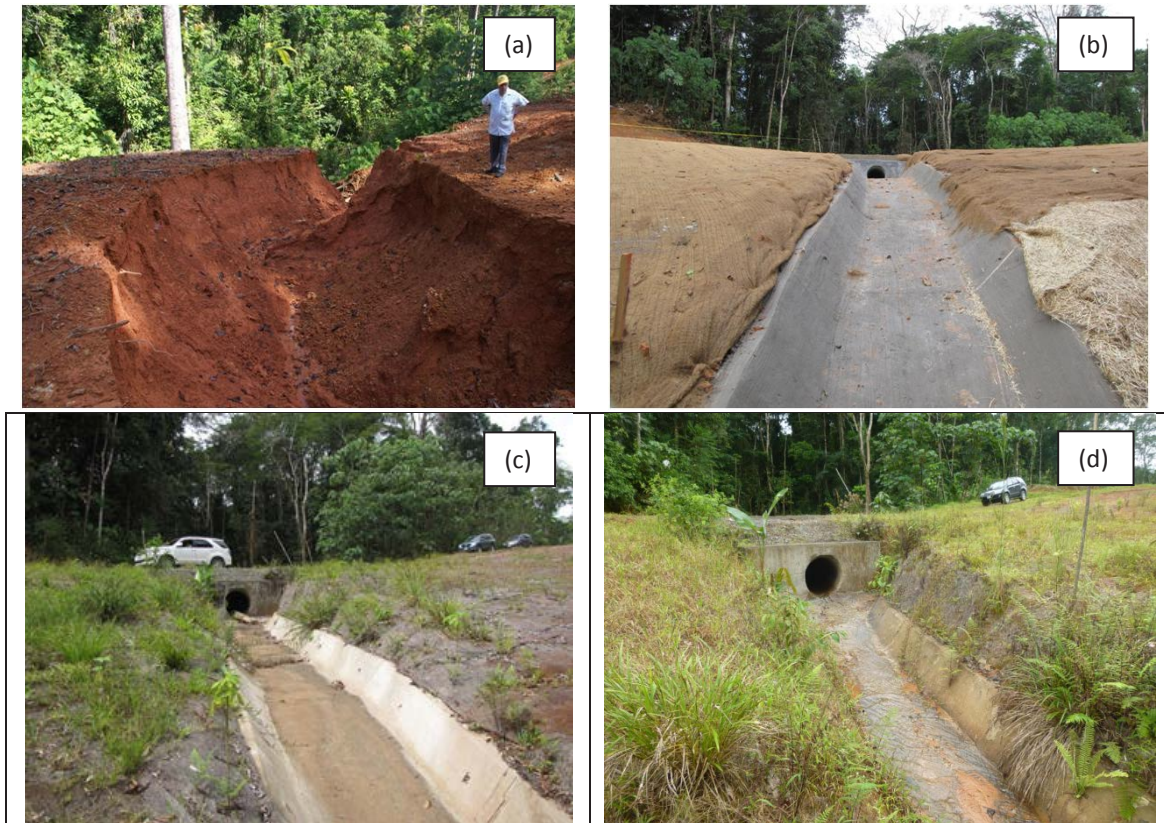
Figure 7.12 View down a large gully in a fill prism created by concentrated runoff from the Road draining to Costa Rican territory to the west of Marker II (a) in February when it was actively eroding and (b) in May when the gully had been back-filled and stabilized using a culvert and concrete drainage channel, with coconut matting used to protect the surrounding fill slope from sheet and rill erosion. Subsequent visits in (c) April and (d) August showed the culverted crossing to be intact after the rainy season and vegetation to be recolonizing the surrounding area. Photographs by the author.
