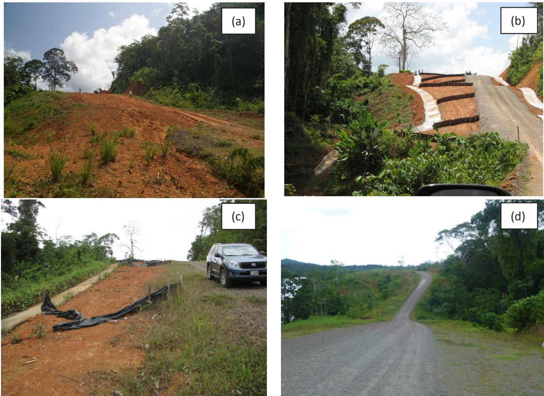
Figure 7.15 Road at East 502480, North 321561, close to the Río Infiernito (a) on 15 February when surface unmanaged runoff from the road bed and surrounding slopes disturbed during construction had caused sheet and rill erosion of bare soil surfaces. (b) The same stretch of road on 7 May 2013 after protection of the road surface using crushed rock, installation of silt fences to prevent sheet and rill erosion while directing down-slope surface runoff into concrete-lined outboard and inboard ditches (c) in April silt fences were showing wear and tear, but vegetation was spreading fast and by August (d) erosion mitigation had been successful at this site. Photographs by author.
