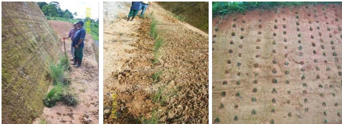
Figure 7.1 Examples of slope preparation and planting to provide surface protection by CODEFORSA along the Road between Marker II and Boca San Carlos
