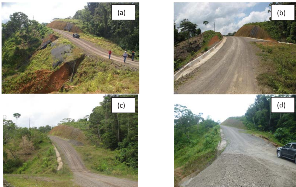
Figure 7.13 Road at East 497867, North 325463 about 6.4 km east of Marker II (a) on 15 February when failure of geotextile slope protection had allowed concentrated out-board runoff from the Road to create two gullies and in-board runoff was undercutting a cut slope (b) on 7 May 2013 after construction of concrete-lined out-board and in board ditches (c) and (d) in 2014 erosion has been effectively mitigated, the gullies have healed and both cut and fill slopes are revegetating. Photographs by author.
