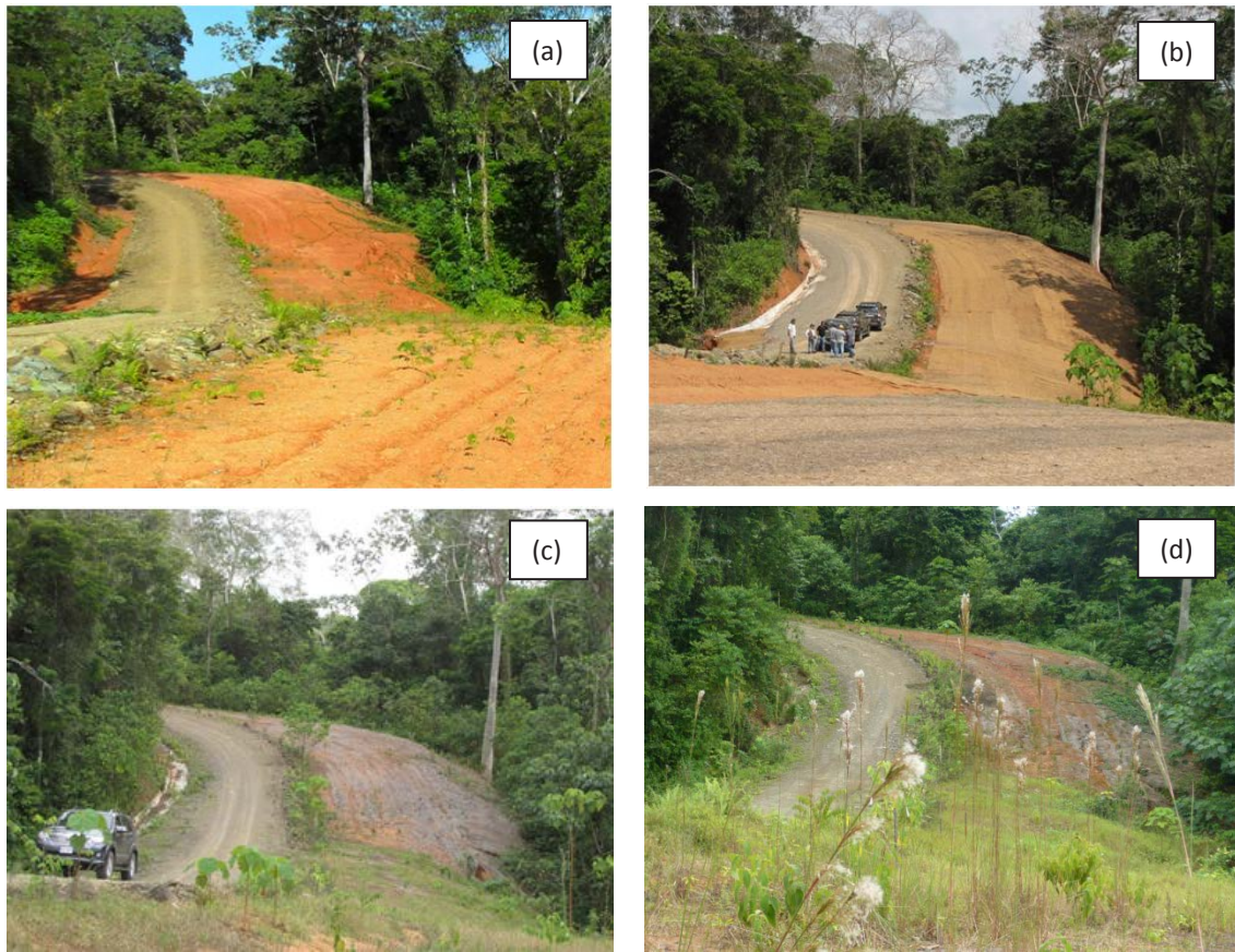
Figure 7.11 The Road near Marker II (a) prior to mitigation work on 15 February 2013 (b) on 7 May 2013 with mitigation measures in place: note in-board drainage channel and extensive biodegradable, erosion control matting (c) on 23 April showing that all mitigation measures survived the rainy season and (d) on 29 August showing that vegetation has stabilized both margins of the road bed and was spreading across the areas protected by coconut matting. Photographs by author.
