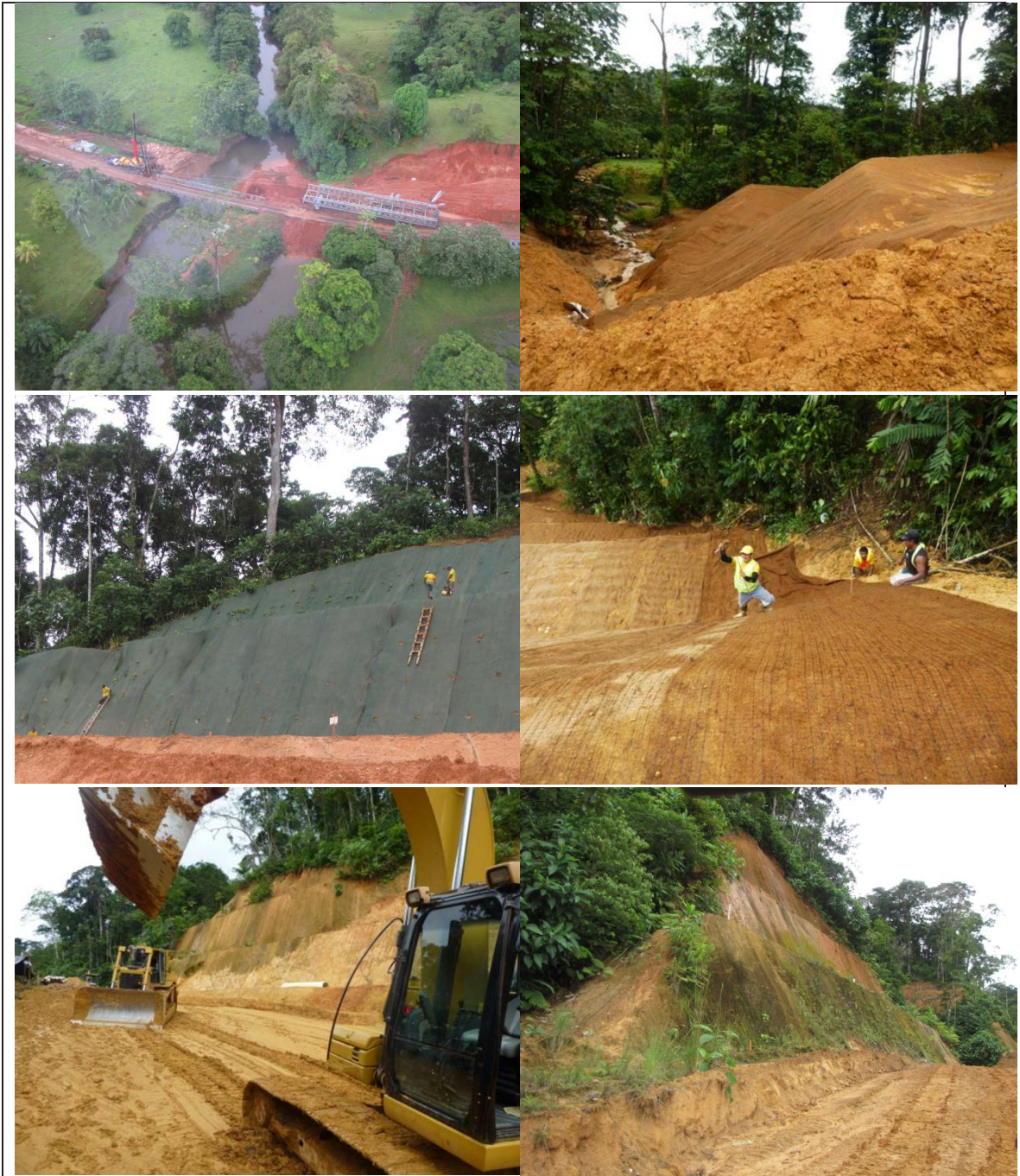
Figure 7.8 Large scale mitigation works by CONAVI on-going at sites around and Caño Cureña, inspected in November 2014. Photographs by author.
