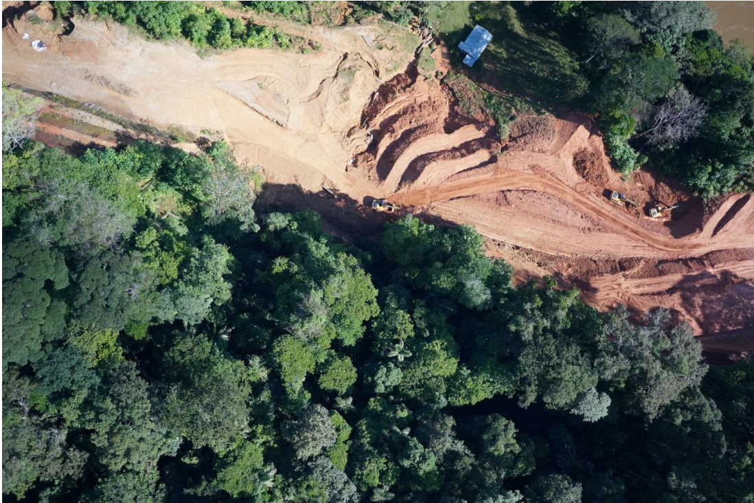
Figure 3. Raw photograph of Route 1856 acquired using an UAV showing on-going mitigation work at slope T-72 (Eroding site 9.6), October 28, 2014.
