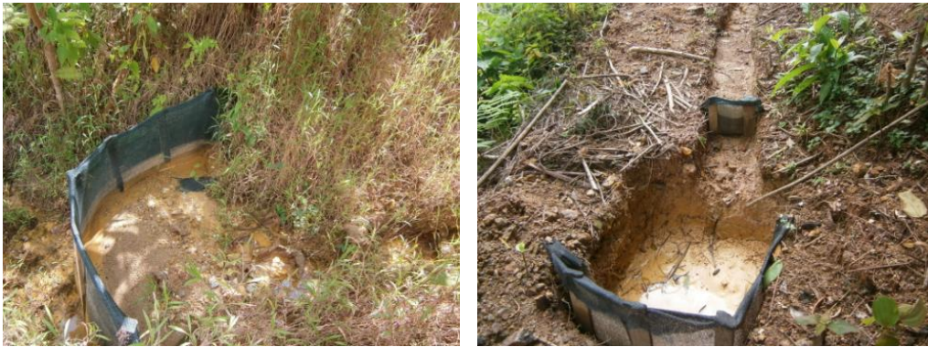
Box sediment traps in gullies and at the end of the drain
