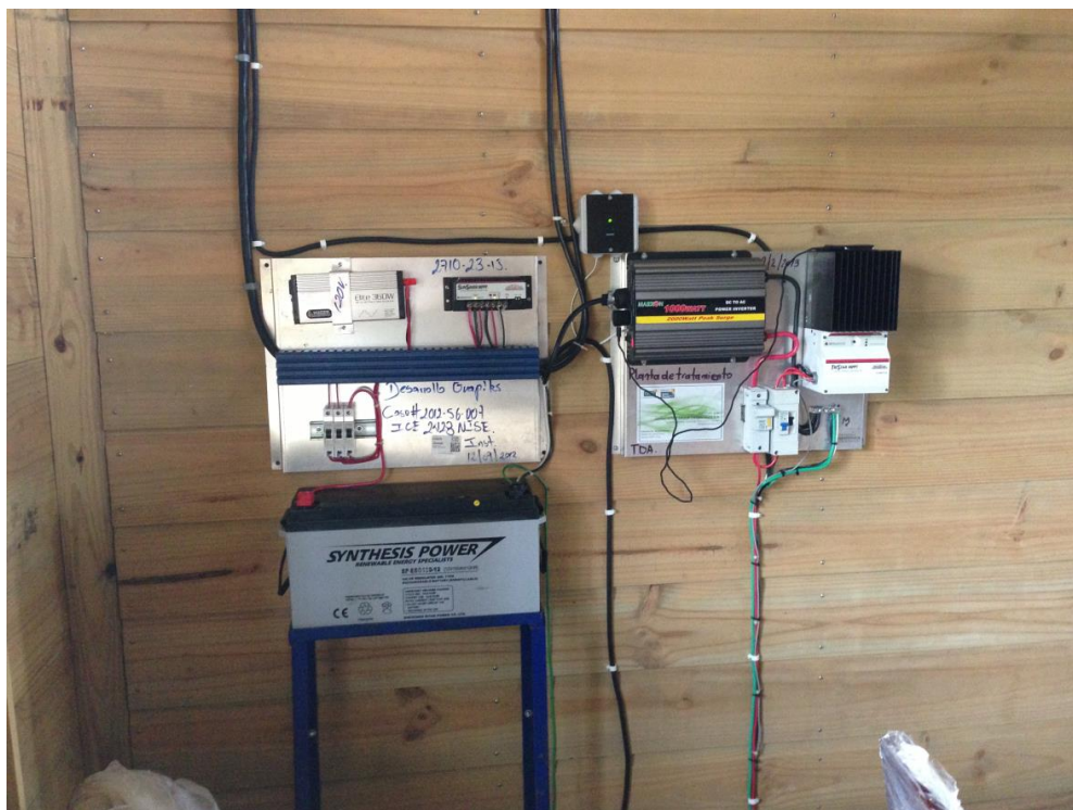
Figure 14: Photovoltaic electric system of the MINAET biological station
