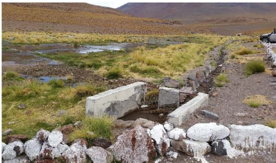
Figure 4 Blocked (and dry) reach of the main canal in zone 3 where the flow has been diverted to a flat wide cross section with manmade obstructions to restore wetland areas.
