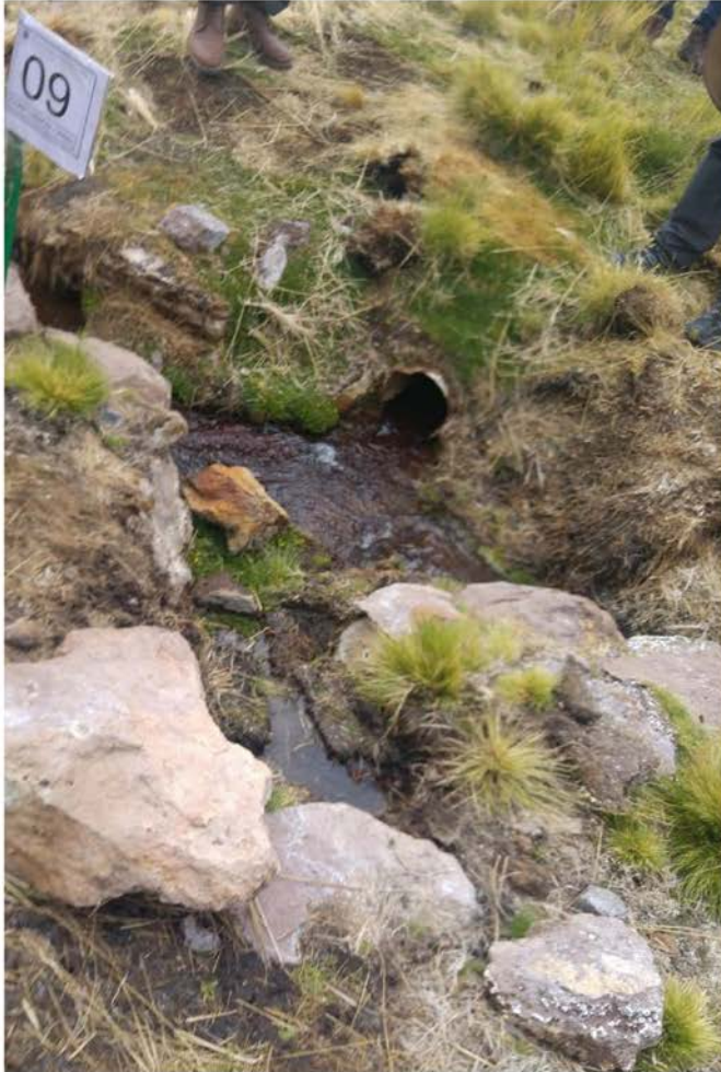
Figure 11 Photo showing drain pipe.
