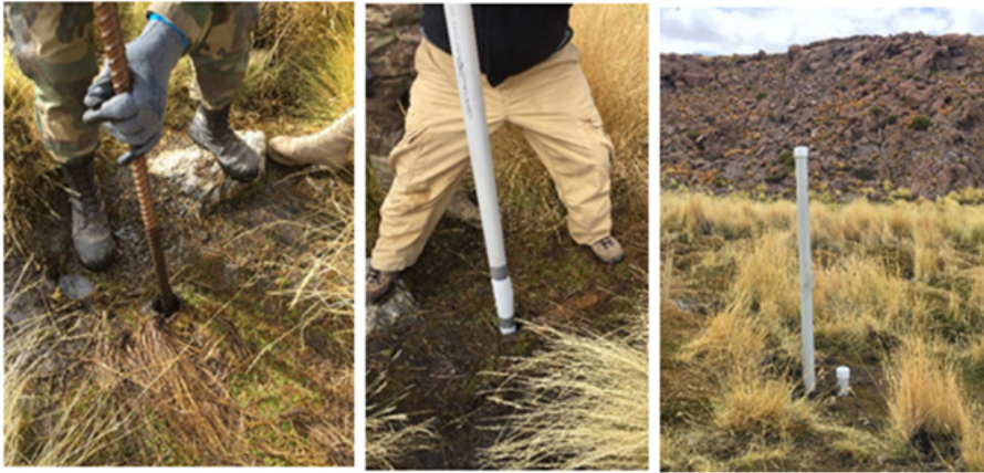
Figure 6. Piezometer installation in the Silala bofedals. Right side: expansion of the hole made with augers. Center: piezometer installation. Left side: site with the two piezometers installed (PN17).
