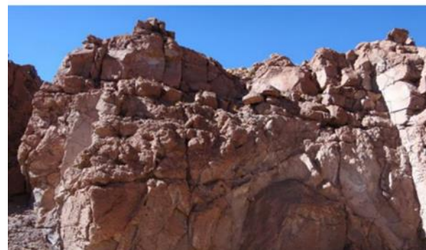
Figure 7-8 Fracturing within ignimbrite walls of the Silala ravine - note the vertical fracture crossing through the section inclusive of varying degrees of welding and lithological variations
