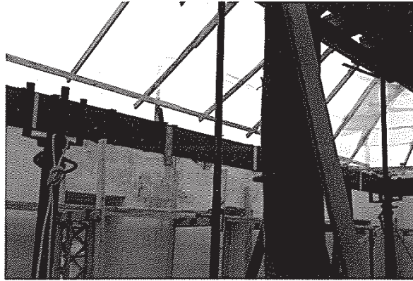
DAMPNESS OF THE WALLS OF THE MOSQUE
