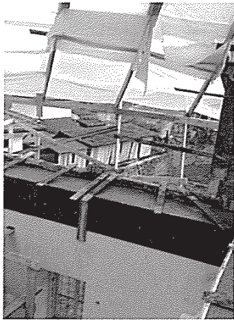
VISIBLE DAMPNESS OF THE WALLS DUE TO PRECIPITATION THROUGH HOLES
