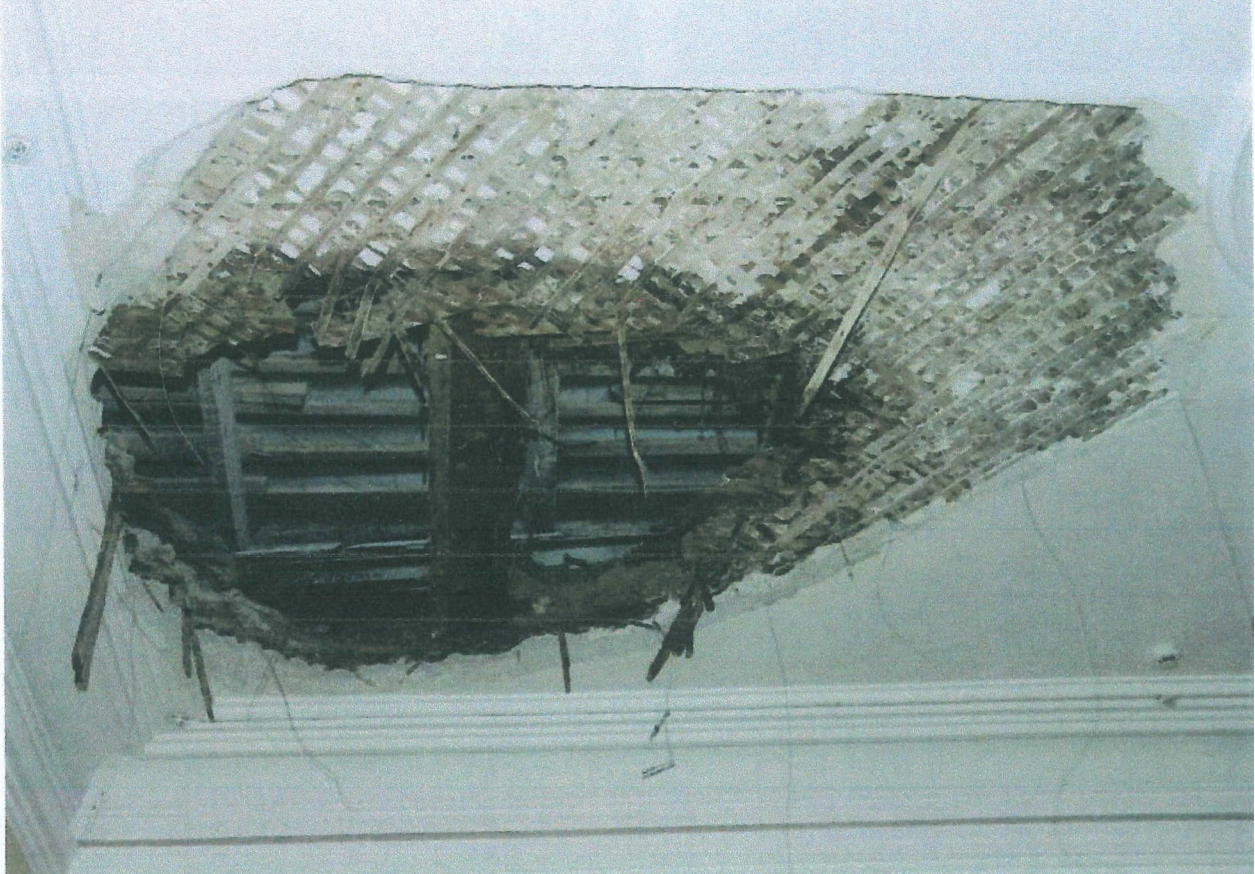
Photo 48. Rot-affected ceiling of the second floor.
