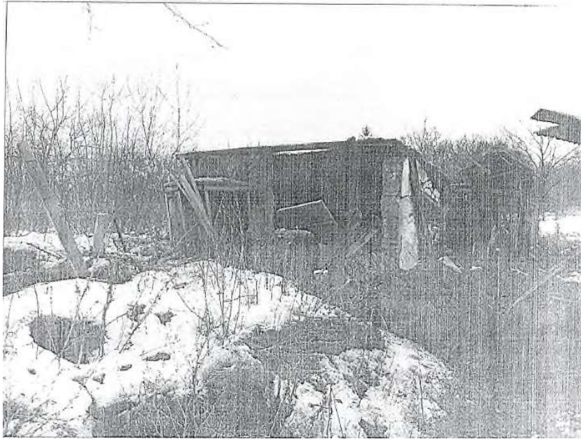
Photo No. 3. The destroyed outbuilding, located behind the residential building.
