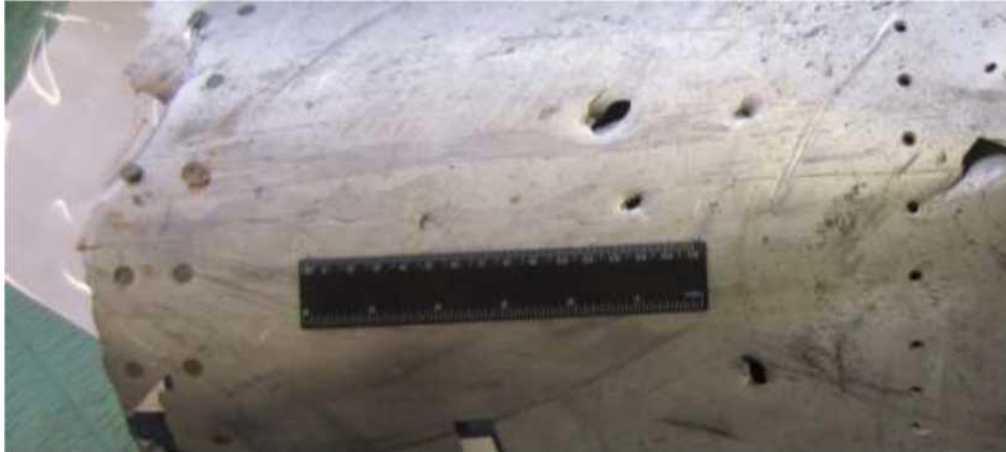
Figure 5.1.53 - Exterior view of fragment of Boeing 777 left wing tip with characteristic damage
