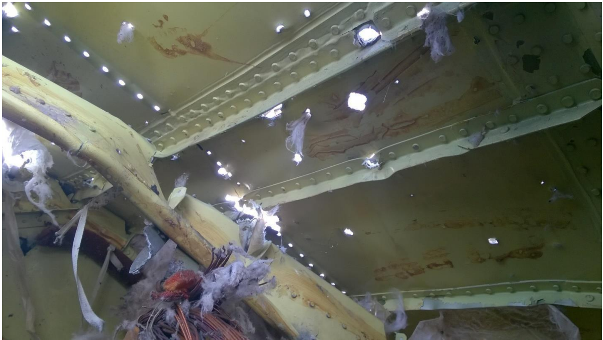
Figure 5.49 - Fragment of upper part of the port (inside view). The fragment shows deformation of the framework elements and detachment of the outer skin from the framework resulting from the detachment of rivet heads
