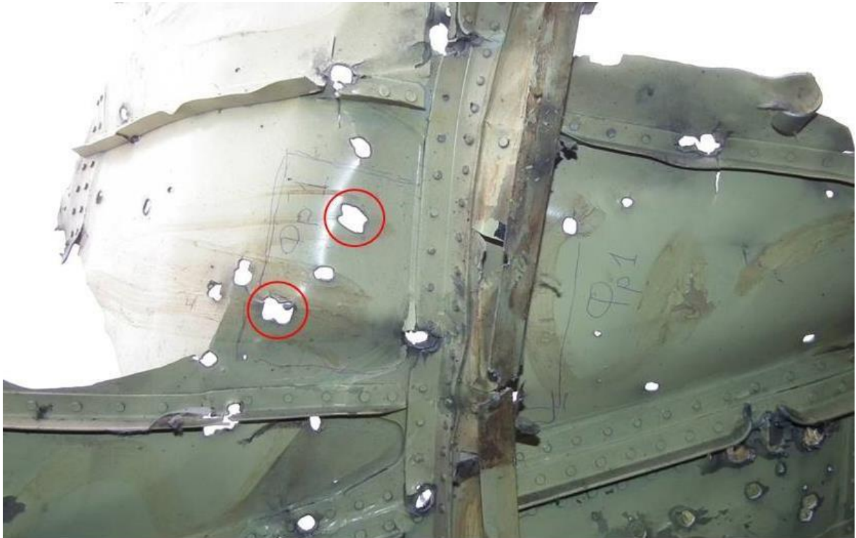
Figure 6.6 - Fragment of the upper section of the port behind the aircraft commander's seat
