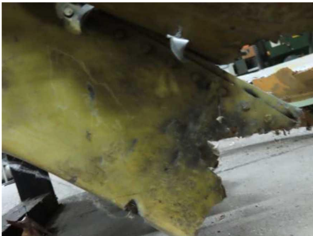
Figure A.3.7 - Perforation, thermal oxidation and deformation of the transverse strength members (bulkheads) resulted in their rupture and subsequent structural failure of the upper port side
