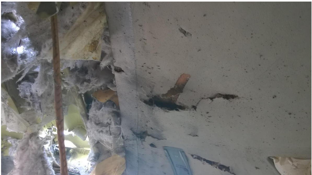
Figure 5.74 - Through-and-through holes in the outer skin and thermal and noise insulation panels on the right side of the cockpit roof (inside view)
