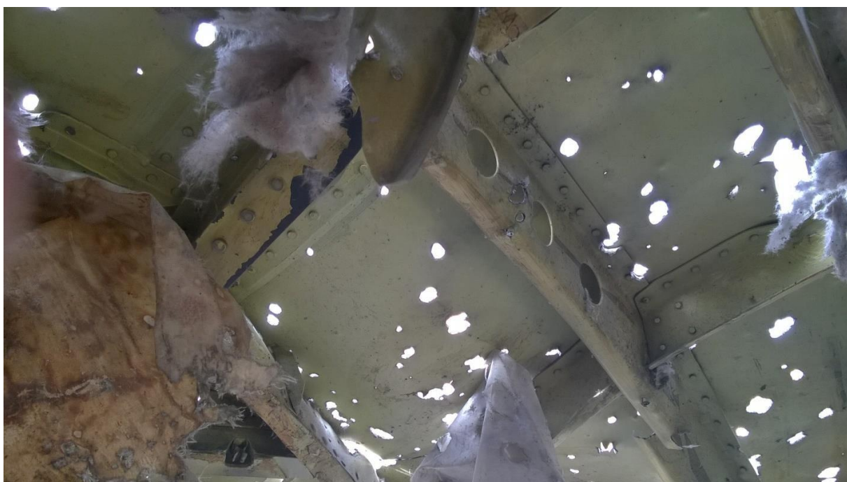
Figure 5.143 - Cockpit roof with through-and-through holes in stringers and signs of damage
