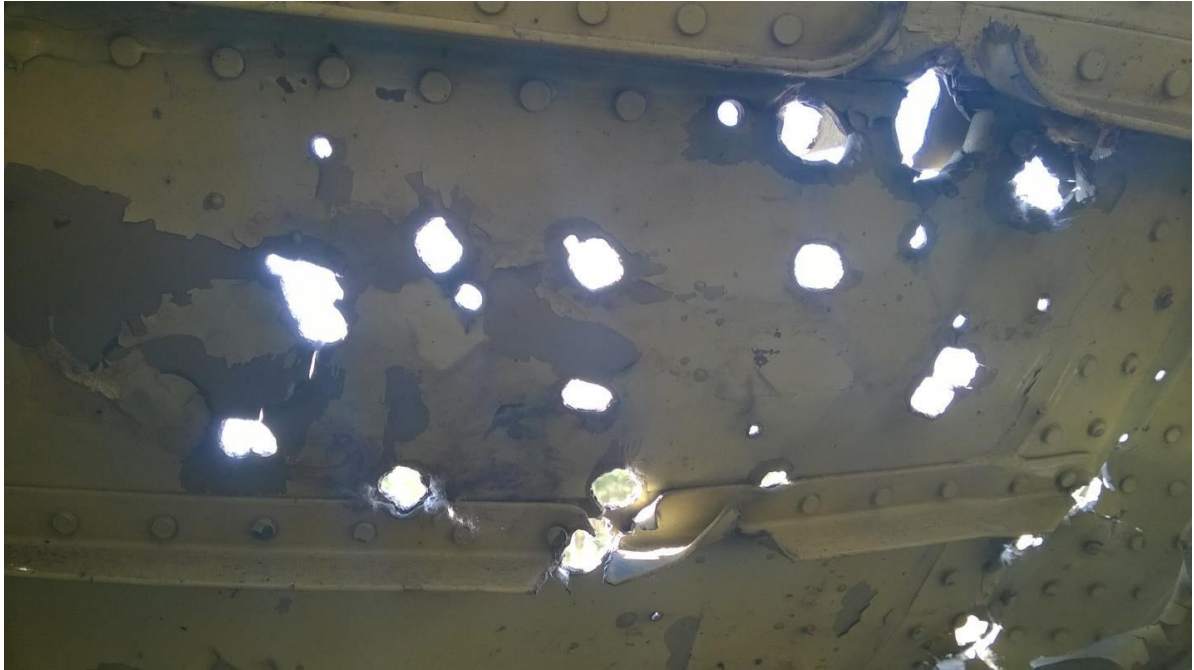
Figure 5.47 - Fragment of the upper part of the port with through-and-through holes caused by ready-made projectiles and missile hull fragments (inside view)
