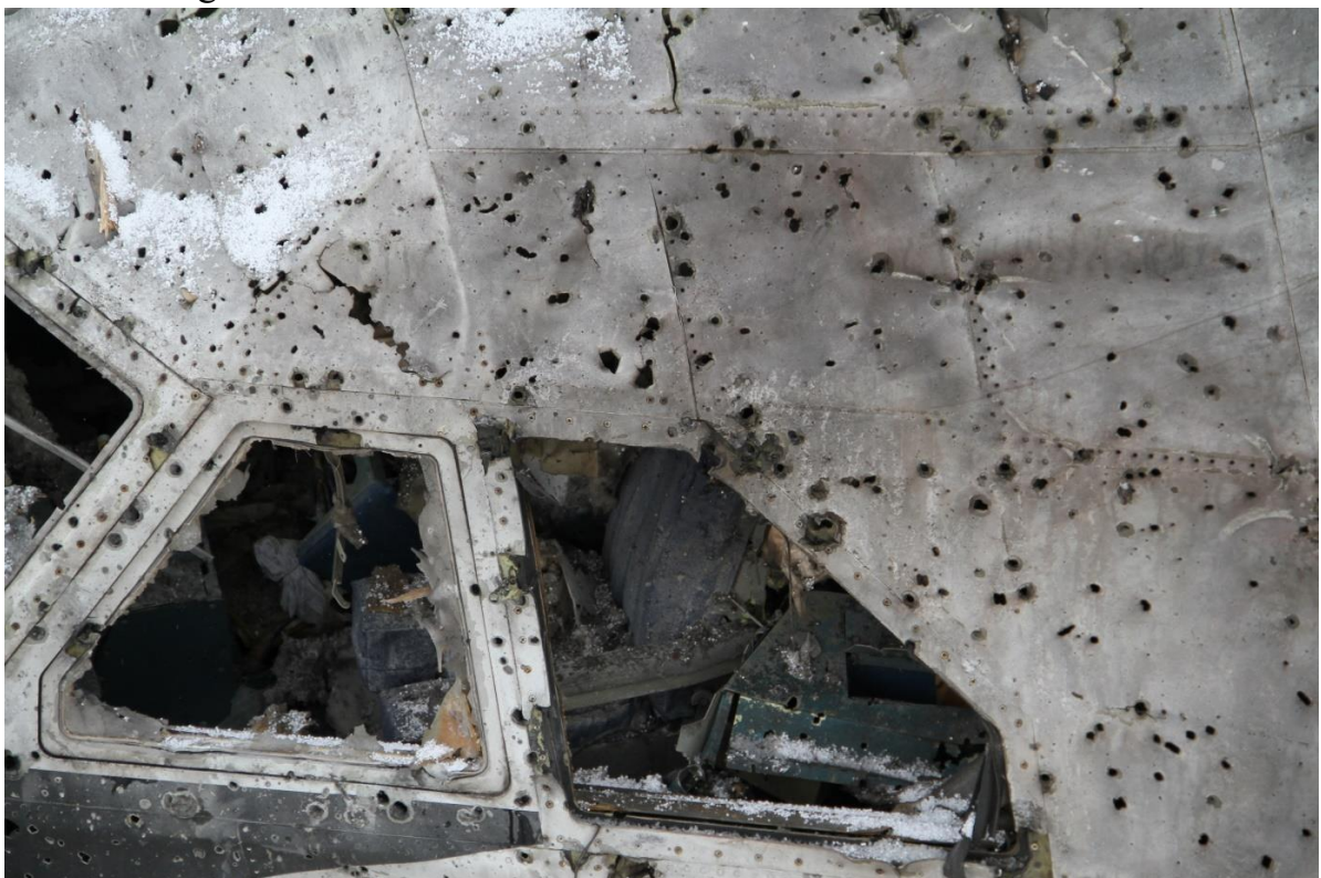
Figure 5.20 - Aircraft commander's second and third windows (top left view)
