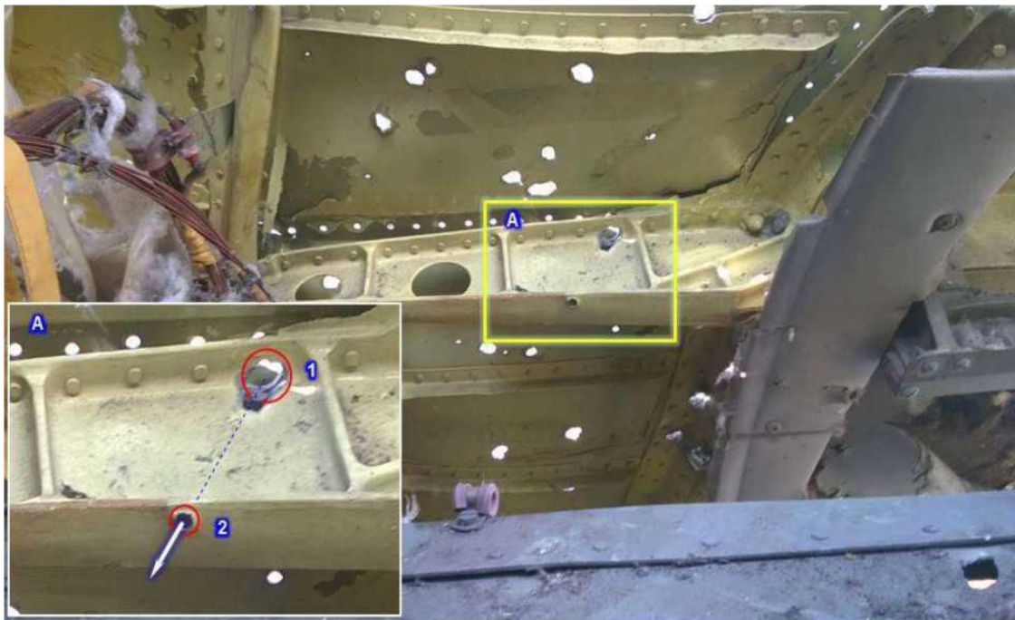
Figure A.4.12 - Through-holes in the outer skin of the port side (1) and in the reinforced stringer of the port side (2)
