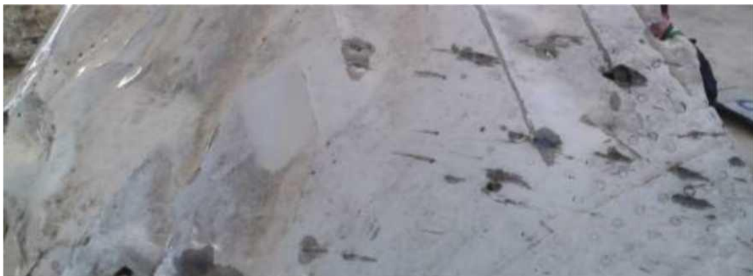
Figure 5.2.1 - Example of characteristic damage near the boundary of the overlapping field on the right side of the cockpit roof
