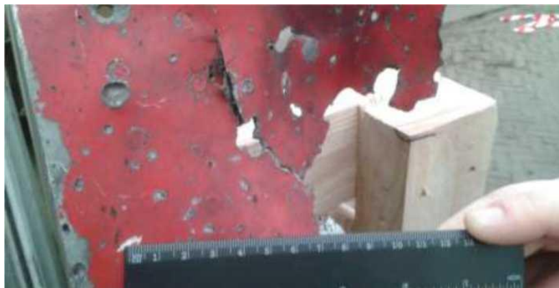
Figure F.14 - Actual through holes, identified as impact damage, located to the right of the bulkhead no closer than 5-10 cm from the level of STA 132.5
