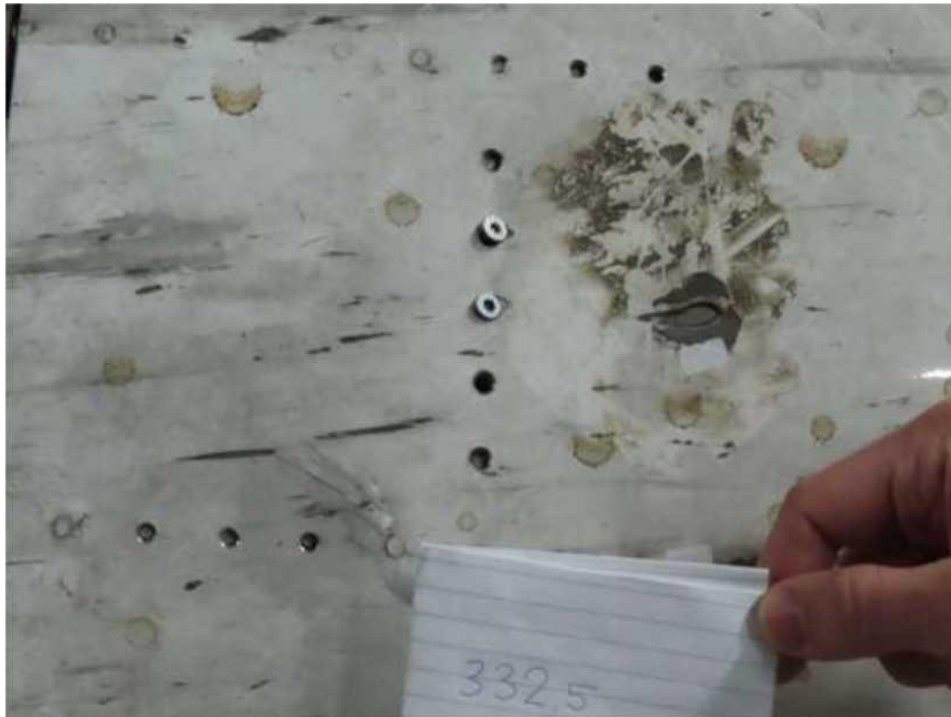
Figure A.1.21 - Example of damage to the outer skin at the edge of the coverage area beyond the level of the STA 332.5 bulkhead
