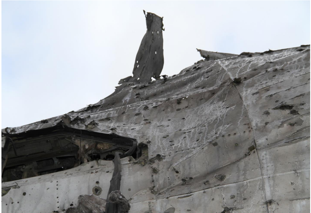
Figure 5.39 - Port side skin showing signs of significant deformation of outer skin in the direction from outside to inside
