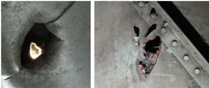
Figure 5.1.57 - Exit "inside-out" through-and-through hole in the structural element of the left engine air intake edge (right). The linear size of the exit hole is about 14 mm
