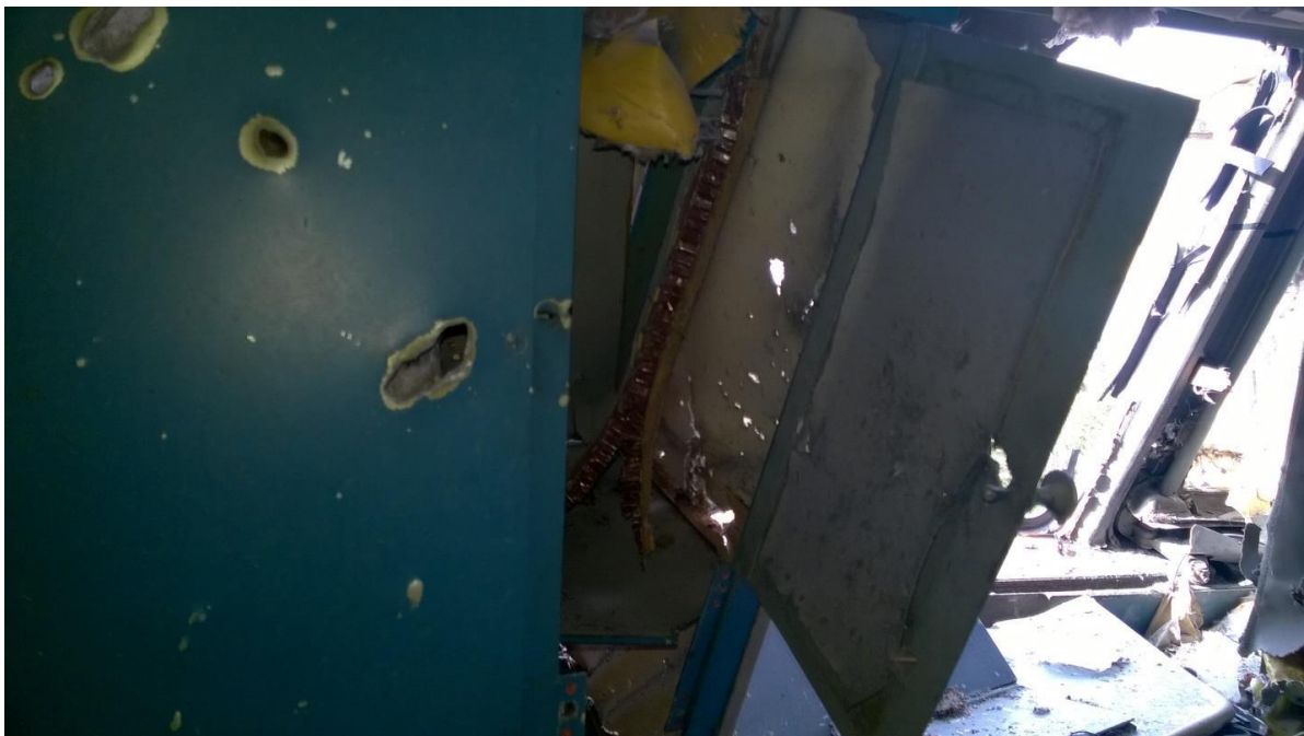
Figure 5.114 - Exit holes in the instrumentation cabinet on the port side (view from the cockpit)
