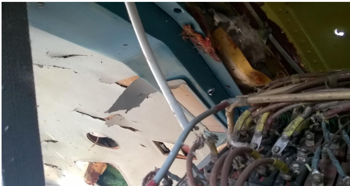
Figure 7.9 - Instrumentation cabinet panel at the top of the starboard side behind the co-pilot's seat. In the upper right-hand corner is an exit hole in the right section of the cockpit roof
