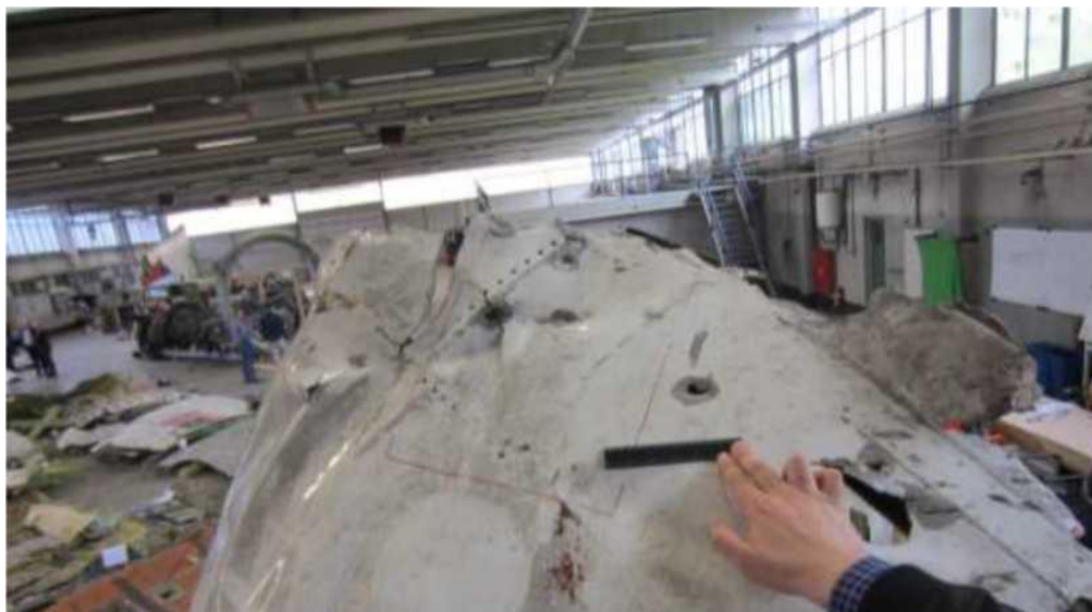
Figure 5.1.19 - Boundary damage in the upper part of the fragment of the right side of the cockpit
