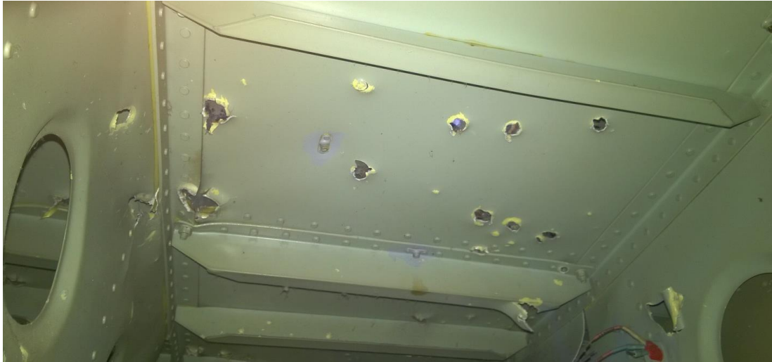
Figure 7.8 - Through-and-through holes in the cockpit floor (bottom view)
