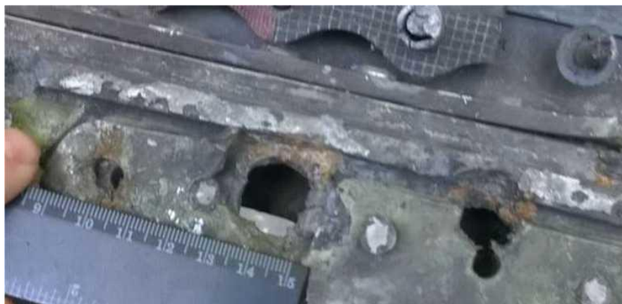
Figure G.4.6 - Entry hole in the structural member has a linear dimension of about 14 mm
