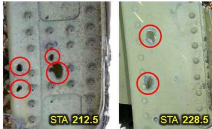
Figure 5.1.42 - Holes in bulkheads STA 212.5 and STA 228.5 are beyond the lower boundary of the fragmentation field on the outer skin
