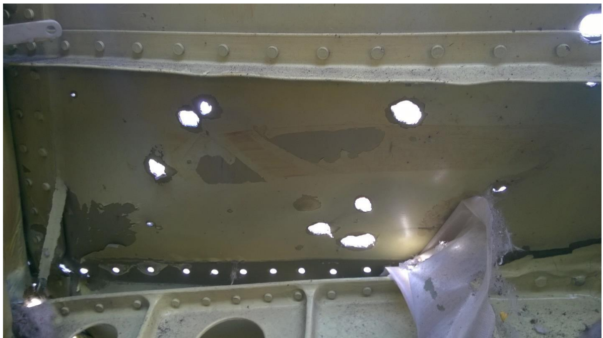
Figure 5.50 - Fragment of the port side behind the aircraft commander's seat (close-up, inside view)
