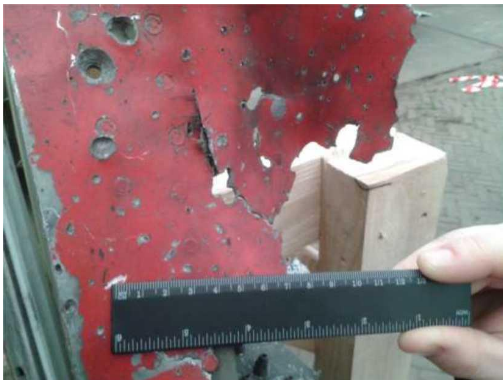
Figure 5.1.11 - Through-and-through holes identifiable as impact damage are located on the left side behind the bulkhead. Photo shows part of the port side adjacent to the bulkhead, with a clearly distinguishable forward boundary of the penetrating damage area.
