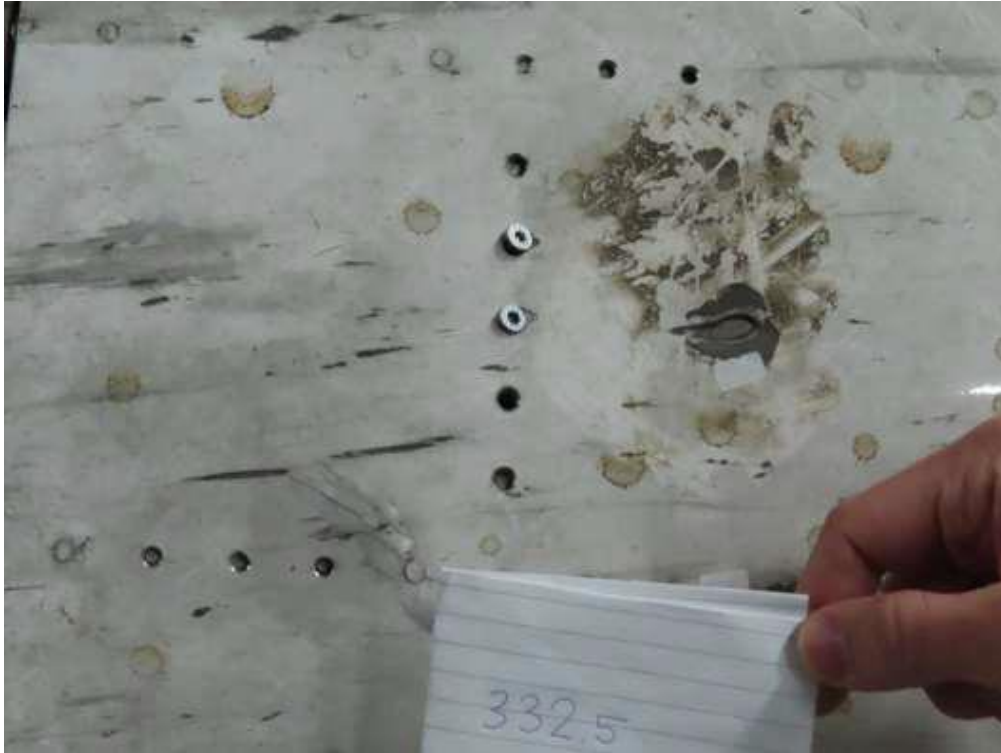
Figure 5.1.23 - Example of damage to the outer skin at the boundary of the cover field beyond the level of the STA 332.5 bulkhead
