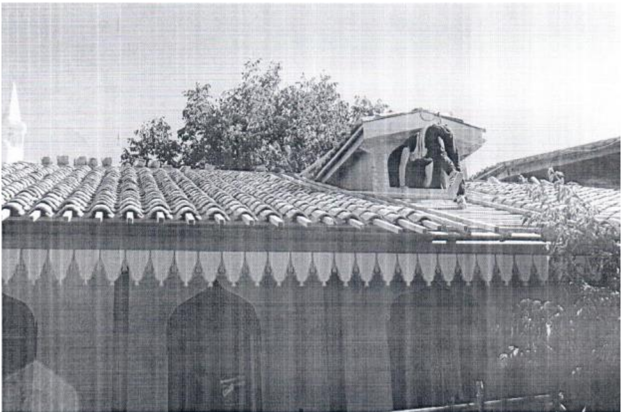
The “Khan’s Palace” Ensemble. Stable Building. Skylight window cladding on the west gable of the roof in axes 4-5. Photo dated 6 October 2022.
