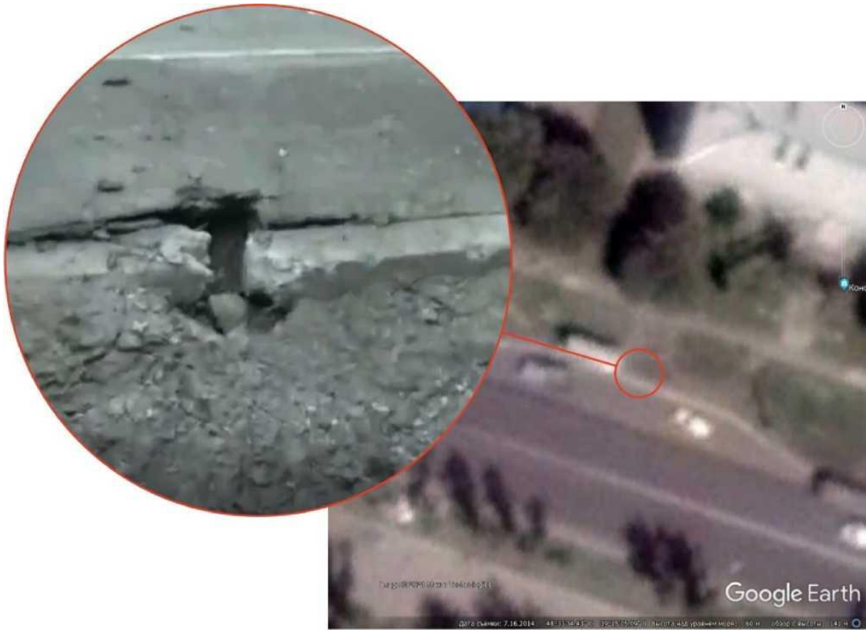
Fig. 43. Hit Instance 10: Shell fragments are traced predominantly on the northern side of the curbstone [44].
