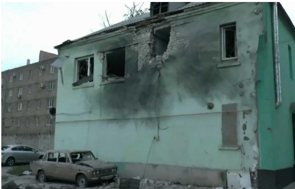
Fig. 17. The hole resulting from the detonation of the shell that hit the northern wall of the two-storey residential building located at 75L Andreyana Linyova Street at the level of the second floor [20].
