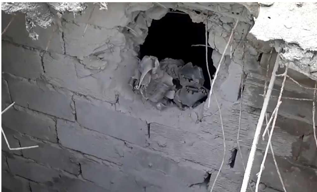
Fig. 26. The hole resulting from the detonation of the shell in the inner wall of the utility structure north of the building located at 75 Andreyva Linyova Street, bldg. 3 [28].
