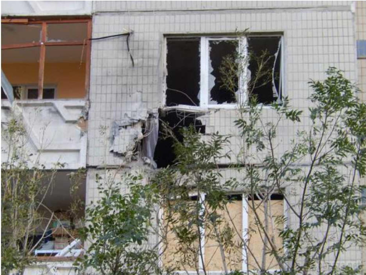
Fig. 7. The northern wall of a multi-storey residential building located at 6 Stepnoy quarter hit by a shell at the level of the fifth floor [10].
