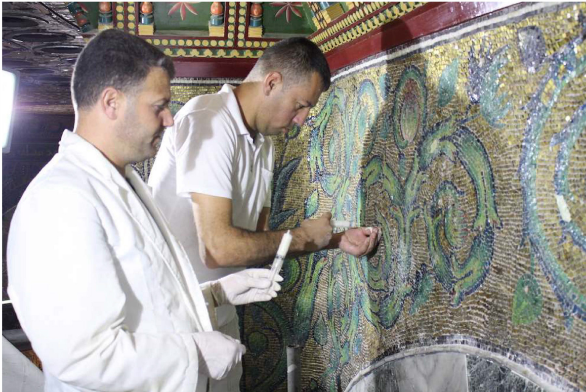
Hashemite Fund Director Dr. Wasfi Kailani and engineer Ra'ef Najem join Awqaf Council members in celebrating the finishing of the 2008-2016 important phase of renovating the mosaic in the Dome of the Rock, July 2016. (Supplied)
