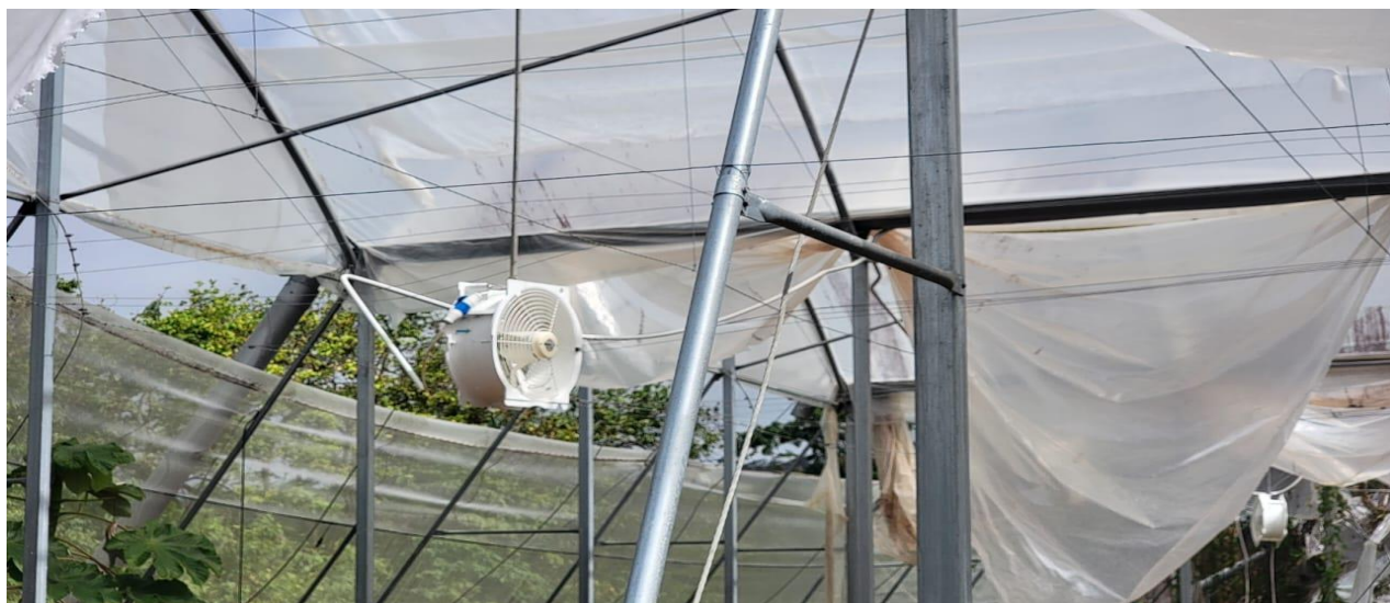
Figure 7: Picture of damaged circulation fans in greenhouse at Mirabeau Station
