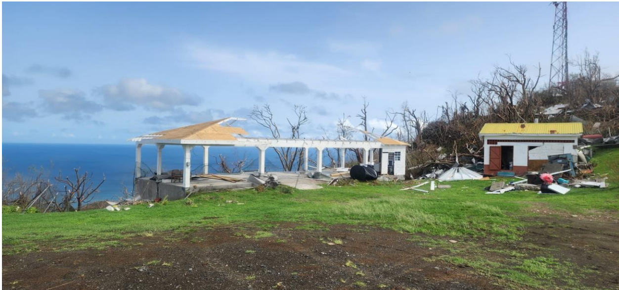
FIGURE 2: DAMAGE TO THE GAZEBO AT PRINCESS ROYAL HOSPITAL. PHOTO: RAM SAHADEO, CDEMA
