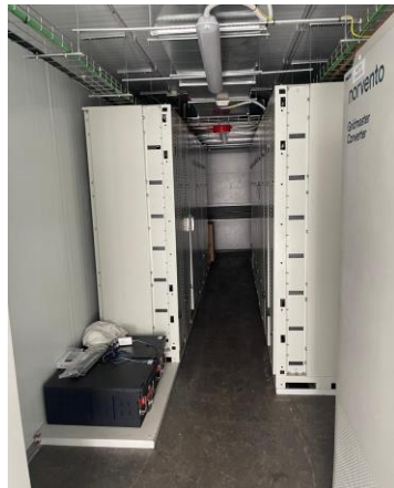
Inside BESS Container
