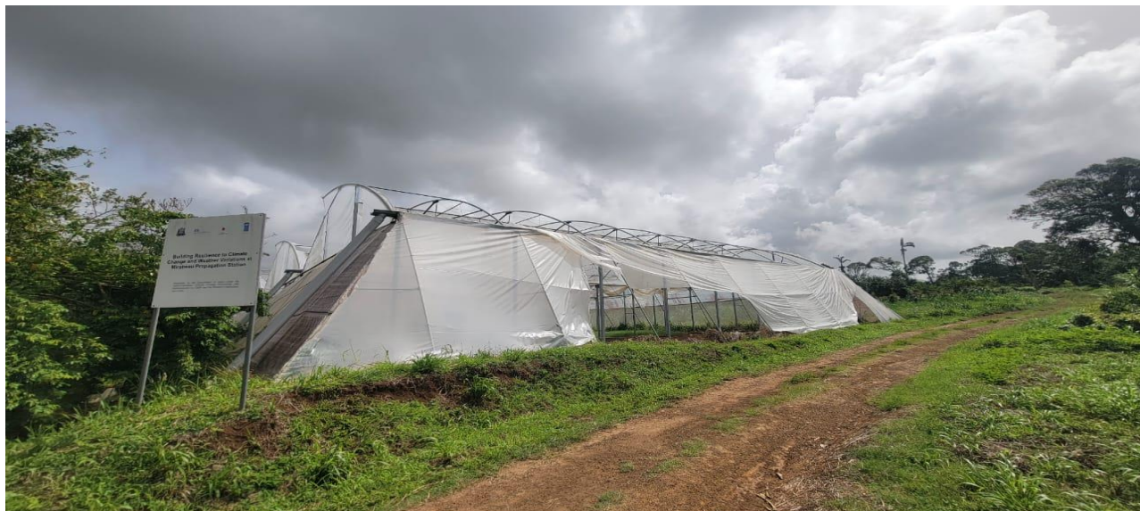
Figure 6: Picture of damaged to plastic covering on greenhouse at Mirabeau Station
