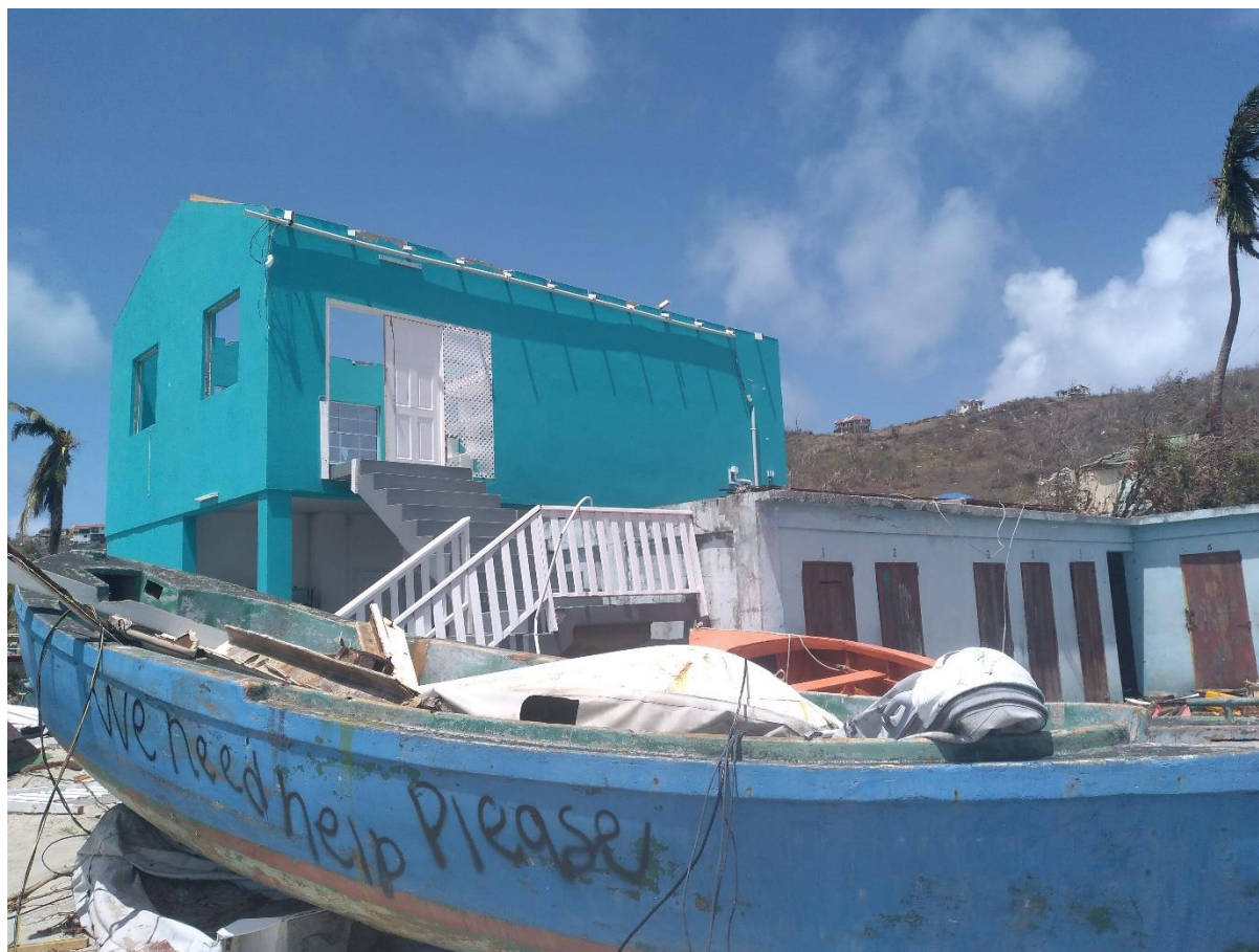
Damaged fishermen co-operative building at Petite Martinique
