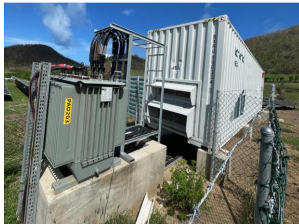
Transformer and BESS Container
