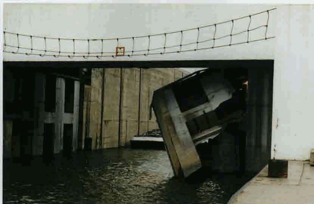
Plate 14a Damaged Lock Gate. Gabčíkovo, 22 March 1994
